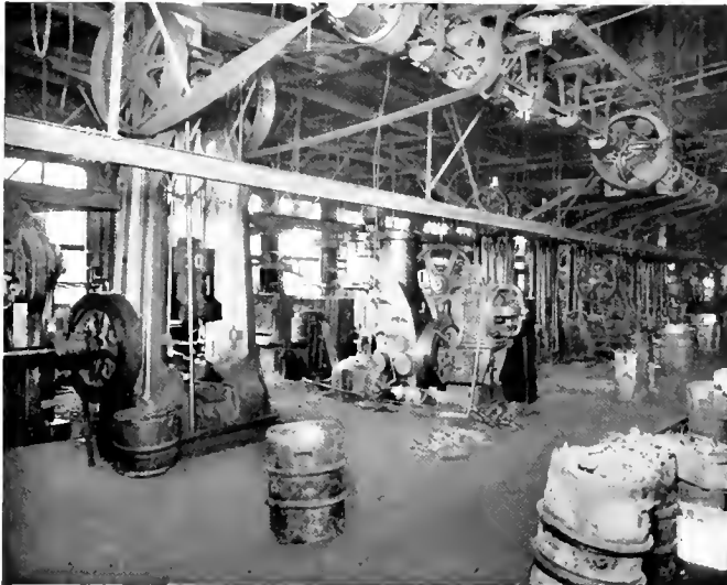
Fig. 4. Group of Nine Drop Hammers consisting of one 2500, two 1600, two 800, two 600 and two 400-lb. hammers, driven from 80 ft. of shafting carrying 18, 30 in. by 8 in. flywheel pulleys and driven by a direct connected 40 h.p. motor. In the middle foreground will be seen a motor-driven air hammer
