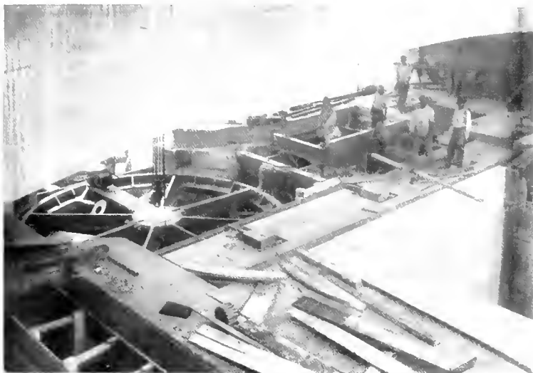
Fig. 6. Miraflores Lower Locks. Miter Gate Moving Machine No. 127. Machine installed complete except short arm and anchor casting on gate leaf. Installation of structural steel in decking commenced. June 20, 1913
