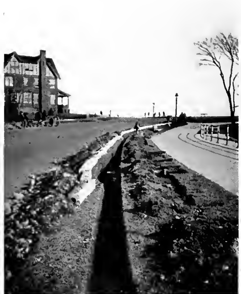
Fig. 2. View showing the Laying of the Ducts through which the Luminous Arc Lamps are Supplied with Current
