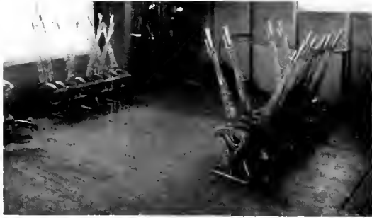
Fig. 6. Operating Levers in Winch Room
