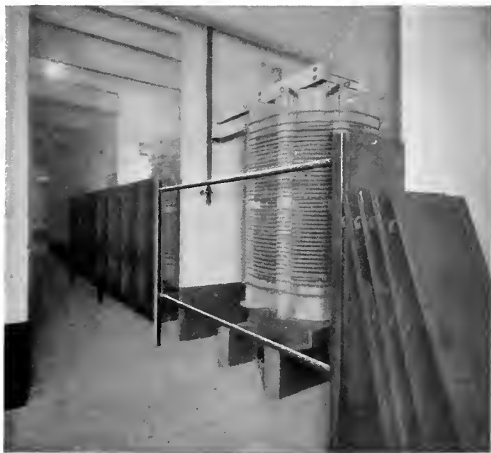
Fig. 17. Reactance Coils in Low Tension Switch Room
