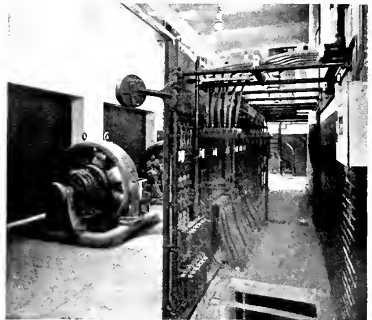
Fig. 11. Back View of the Synchronous Converter Switchboard (Front View, Fig. 16)
