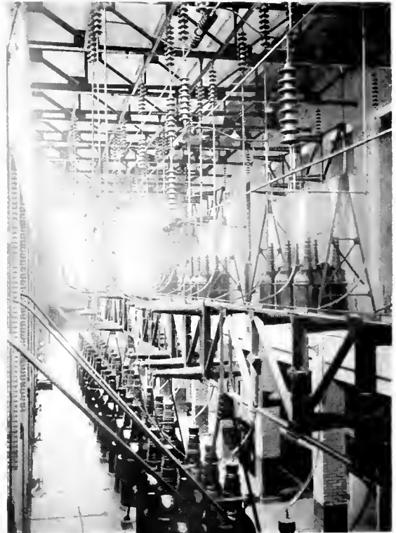
Fig. 32. High Tension Oil Switch Gallery St. Louis Substation
