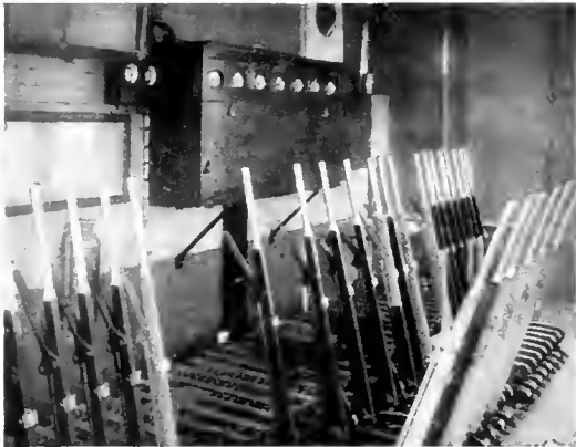
Fig. 8. Mechanical Interlocking Machine with A.C. Electric Locks. A-C. Indicator on Wall
