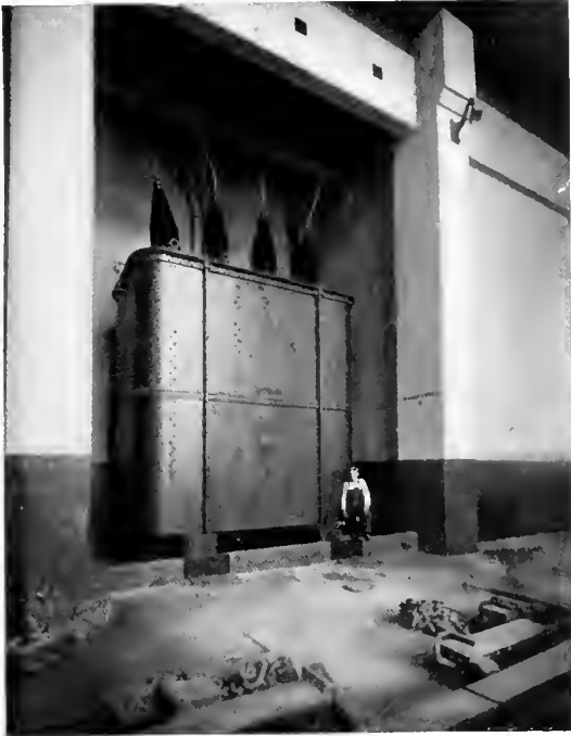
Fig. 14. 9000 Kv-a. Transformer. June 3, 1913
