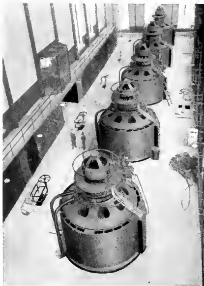
Fig. 10. Five of the 10,000 Kv-a. Main Generating Units
