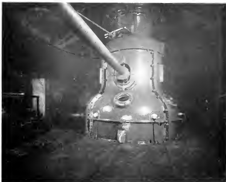
Fig. 11. Step Bearing for Unit No. 1
