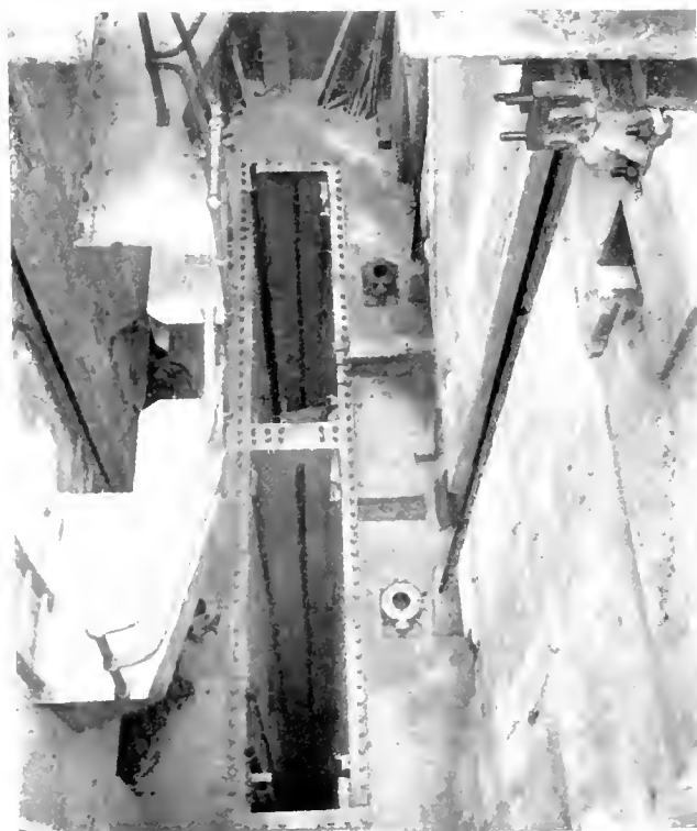
Fig. 3. Miraflores Lower Locks. Rising Stem Gate Valve Machinery Chamber Nos. 442 and 443, West Side Wall. All anchor bolts set in concrete with bulkhead frame, guide rails, screws, bearings, wall brackets and subbase in place. July 18, 1913
