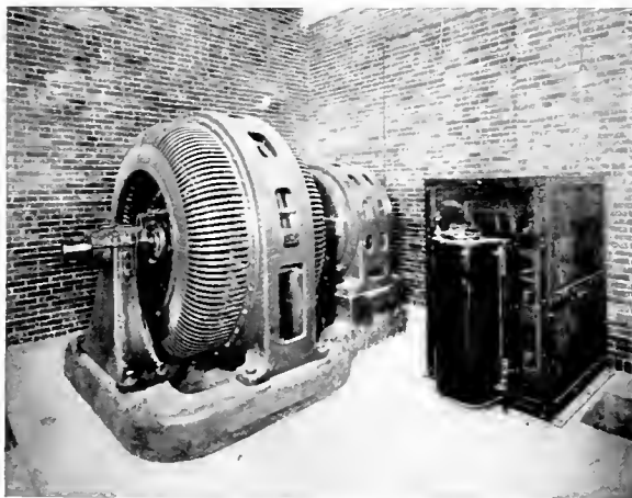
Fig. 12. 835 Kv-a. 2300 Volt Sine Wave Generator, and 450 H.P., 440 Volt Motor. United Electric Light and Power Company, New York City
