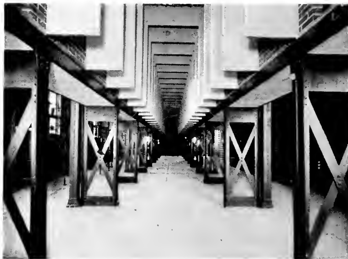
Fig. 14. Duplicate 33,000-Volt Bus Structure showing Transite Barriers
