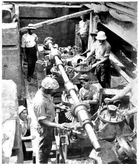
Fig. 2. Miraflores Upper Locks, Rising Stem Gate Valve Machine. June 10, 1913
