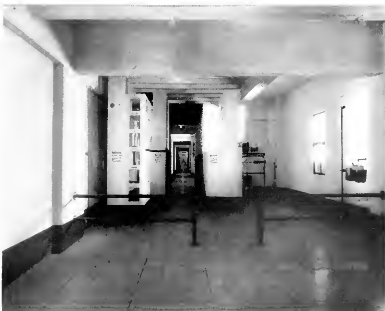
Fig. 20. Looking South Through Low Tension Bus Room
