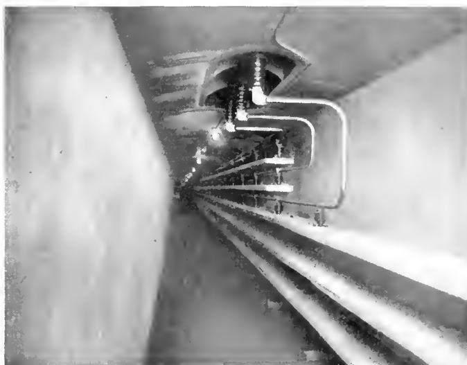
Fig. 15. Low Tension Bus Bar Compartments in Tunnel
