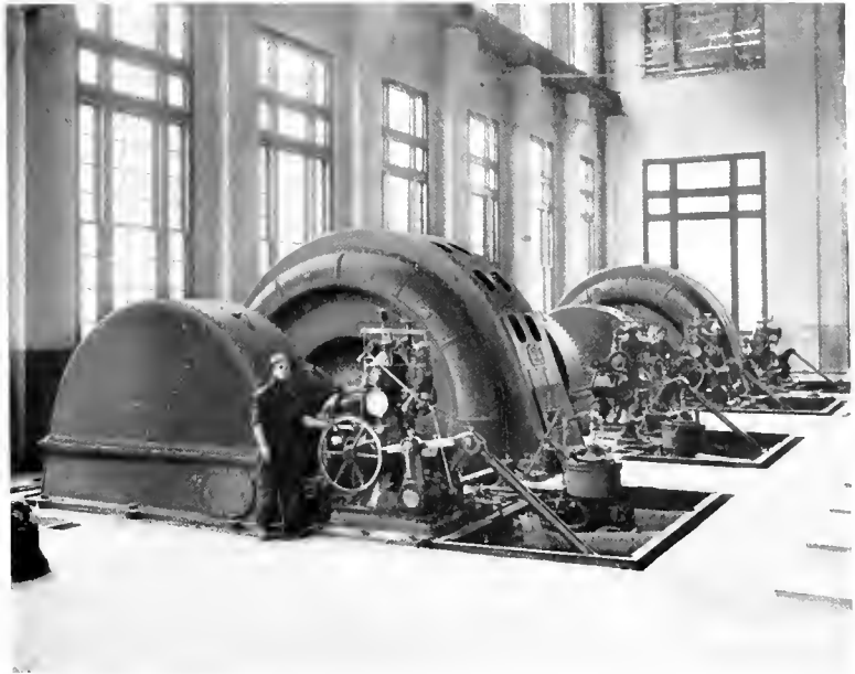
Fig. 3. 17,500 Kv-a. Generators, Big Creek Development, Pacific Electric Light & Power Company
