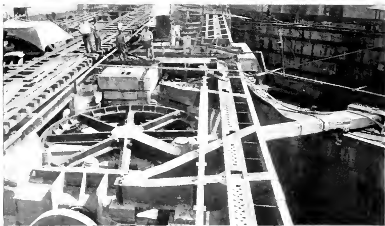
Fig. 5 Gatun Upper Locks. Miter Gate Moving Machine; Structural Steel Girders for towing locomotive track supports in foreground. June, 1912
