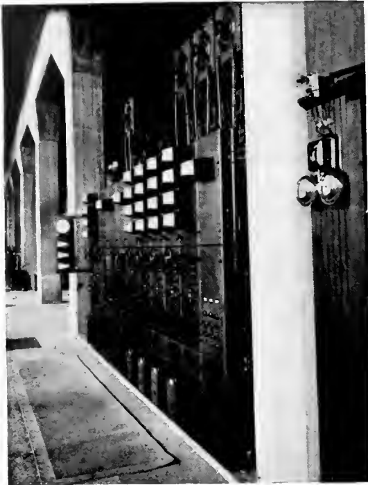
Fig. 4. Front View of Switchboard Installed at Power House
