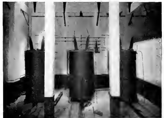
Fig. 12. 10,000 Kv-a. Transformer Bank
