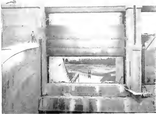
Fig. 8. Gatun Spillway Gate. One complete gate with operating mechanism. Looking downstream, with gate partly open. July 15, 1913
