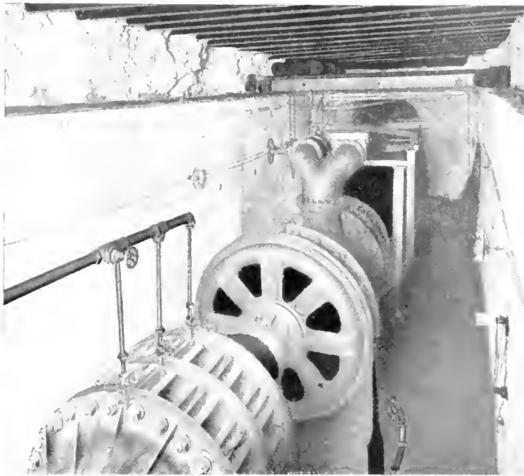
Fig. 3. 1000 h.p. 2300 Volt 720 r.p.m. Induction Motor Direct Connected to 5000 g.p.m. Six-stage Centrifugal Pump Operating Against 500 Ft. Head, Located at Hampton Water Shed Sump. D., L. & W. R. R. Co. Mining Dept.
