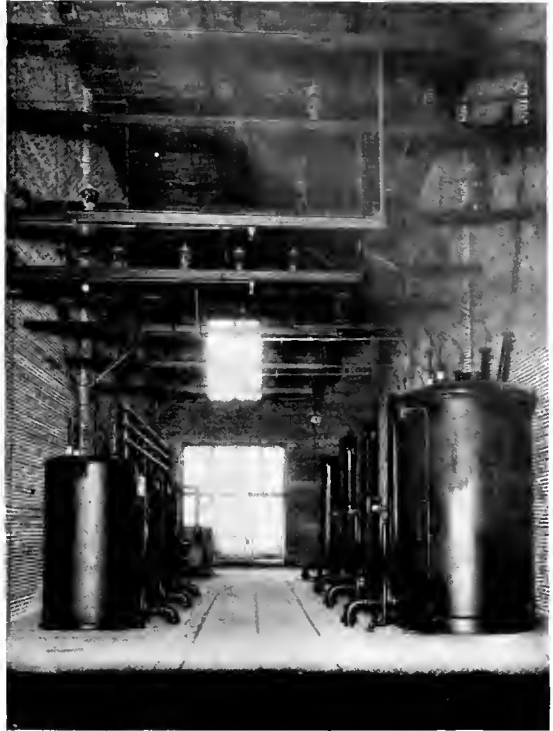
Fig. 12. Transformer Room at the Substation
