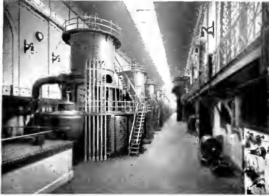
Fig. 4. Interior View of the Fisk Street Station of the Commonwealth Edison Company, Chicago. Approximate Capacity 110,000 Kw.
