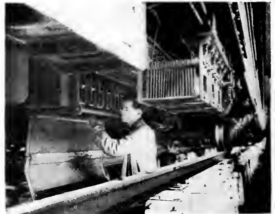
Fig. 2. View of Underbody of Car, Showing Ease with which Resistance Grids and Contactor Box can be Inspected
