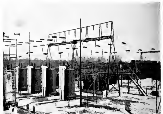
Fig. 3. A View of a Bank of Transformers, Oil Switches and a Lightning Arrester at the Millbury Outdoor Substation
