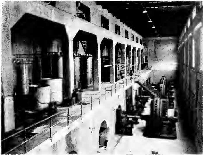
Fig. 2. An Interior View of Power House. Note the Oil-Drying Apparatus in Operation on the Gallery
