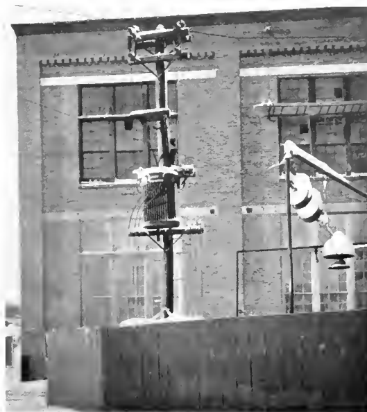
Fig. 13. 25 Kw. Transformer and Switching Equipment after Snow Storm. An Installation for Supplying 110-220 Volt Service from a 16,500 Volt Transmission Line
