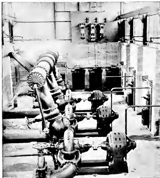
Fig. 2. Direct-connected, Motor-driven Centrifugal Pumps Providing Injection Water for Vacuum Pans and Multiple-Effect Evaporators
