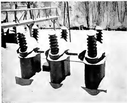
Fig. 4. A View of the Oil Switches at the Millbury Outdoor Substation after a heavy fall of snow
