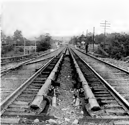
Fig. 7. View of Third Rail Showing Form of Jumpers Used, Oneida Line
