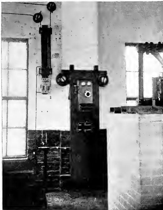
Fig. 4. Front View of the Telephone and Its Protective Equipment as Installed
