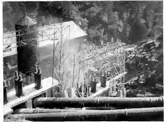
Fig. 15. Lightning Arrester Equipment
