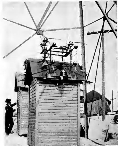
Fig. 3. Telephone Booth Connected, Showing Disconnecting Switch and Horn Gaps
