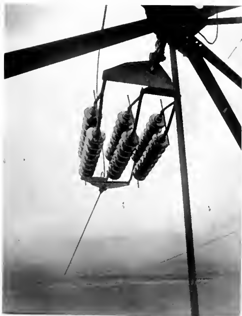
Fig. 29. River-Crossing Insulator on Entrance Structure on Power House Roof
