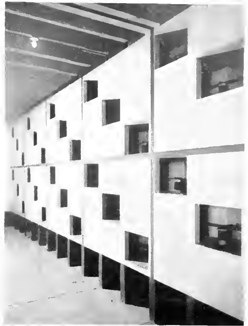
Fig. 21. View of Low Tension Bus Compartments
