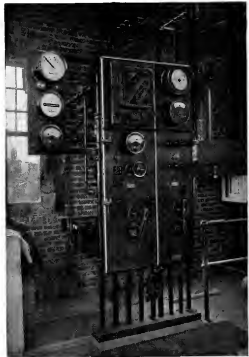
Fig. 6. Railway Signal Power Station Installation, Pennsylvania Railroad
