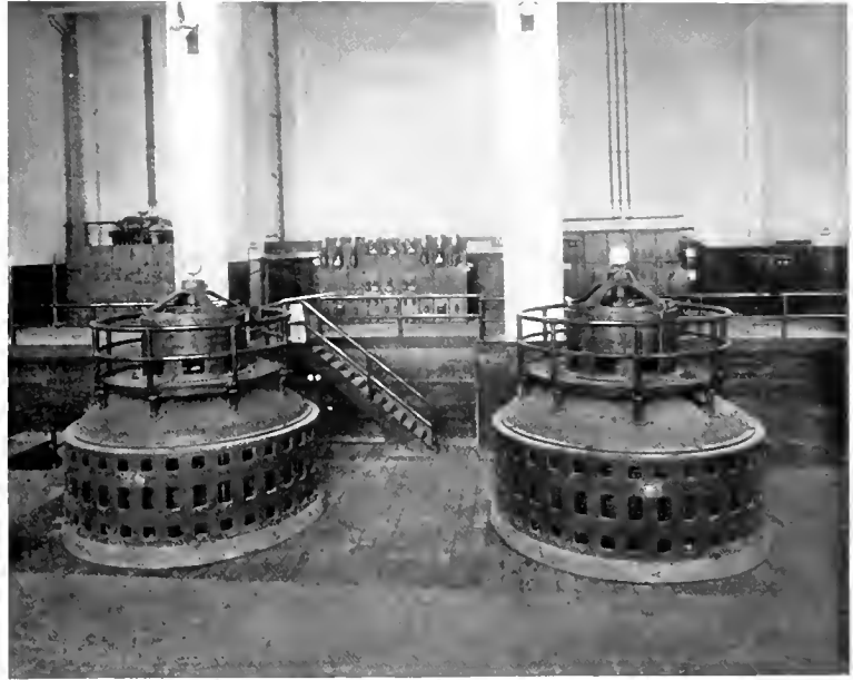
Fig. 12. Auxiliary Alternators Nos. 1 and 2. June 10, 1913
