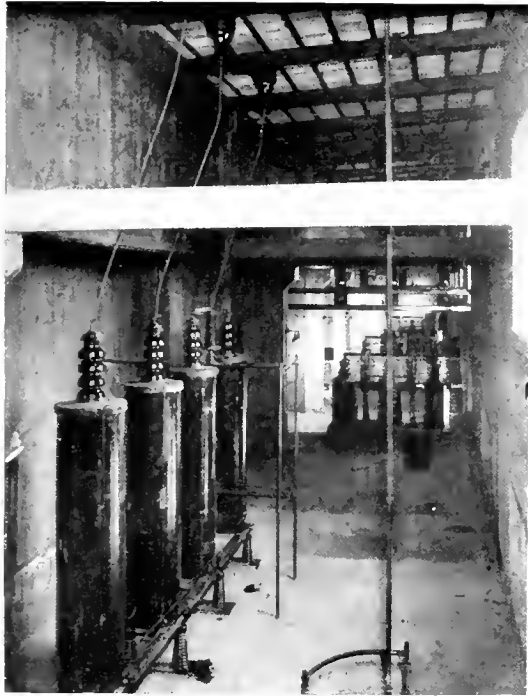
Fig. 6. 66,000-Volt Switches and Lightning Arresters Located at Power House
