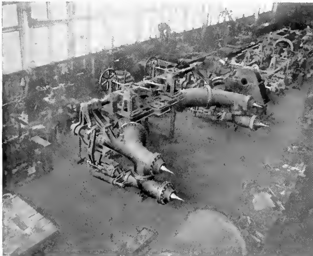
Fig. 3. Excellent example showing application and method of governor and hand control connection for double overhung type Pelton-Doble auxiliary relief needle regulating nozzles
