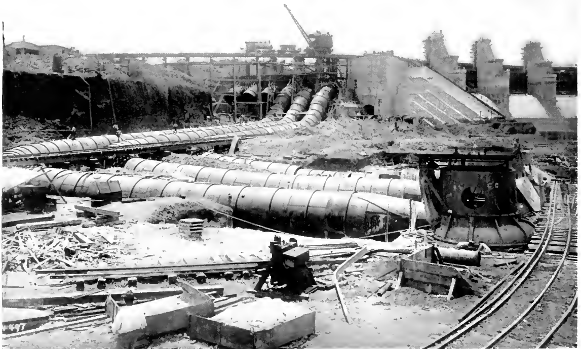
Fig. 2. Left-hand Side of Panoramic View of Gatun Hydro-Electric Installation under Construction, showing Pipelines and Turbines Erected
