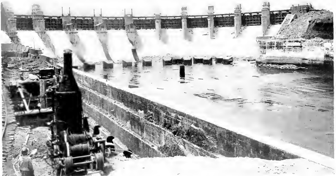
Fig. 4. Right-hand side of Panoramic View of Gatun Hydro-Electric Installation under Construction, showing Ogee Spillway Dam
