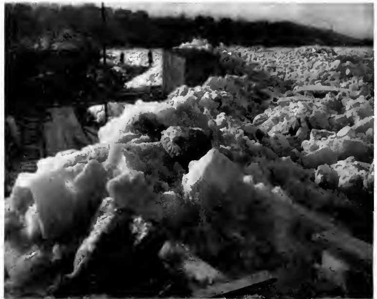
Fig. 2. Timber Cofferdam for Power House Resisting Ice Jam. March 24, 1912. Cofferdam 25\frac{1}{2} feet high
