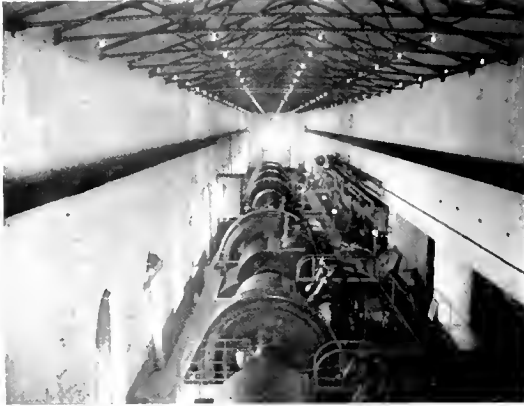
Fig. 10. Interior View Lake Buntzen No. 1 Power House, B. C. Electric Railway Company, Ltd., of Vancouver, B. C., showing a number of high capacity Pelton-Doble Tangential Waterwheel Units of modern design
