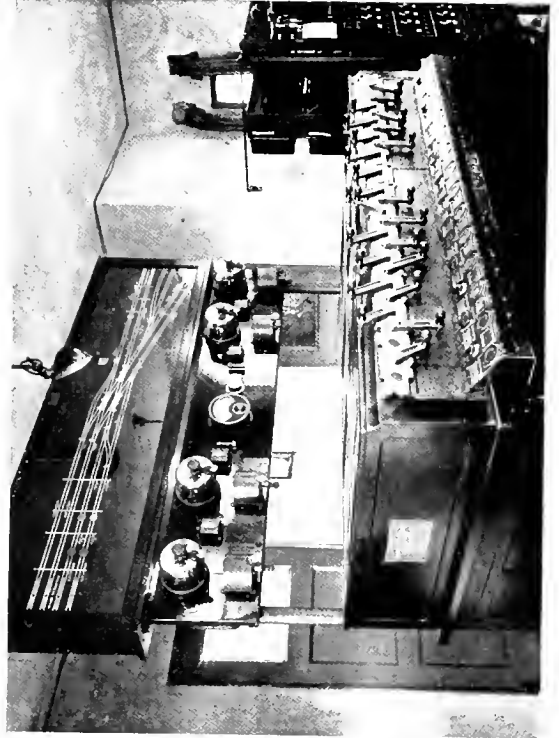
Fig. 13. All-Electric Interlocking Machine, New York, Westchester & Boston Railroad, Columbus Avenue Tower
