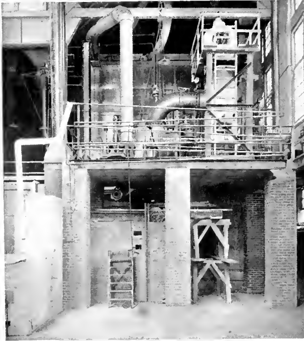
Fig. 7. Mercury Boiler and Turbine as Erected in Power House
