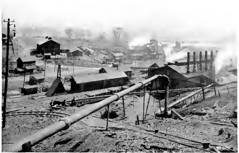
Fig. 1. An Example of what Distribution of Power by Steam means. Note the long line of exposed pipes
