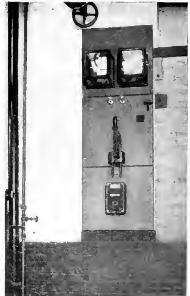
Fig. 2. Control Board, Showing Operating Lever of the Oil Switch and the Curve-drawing Instruments
