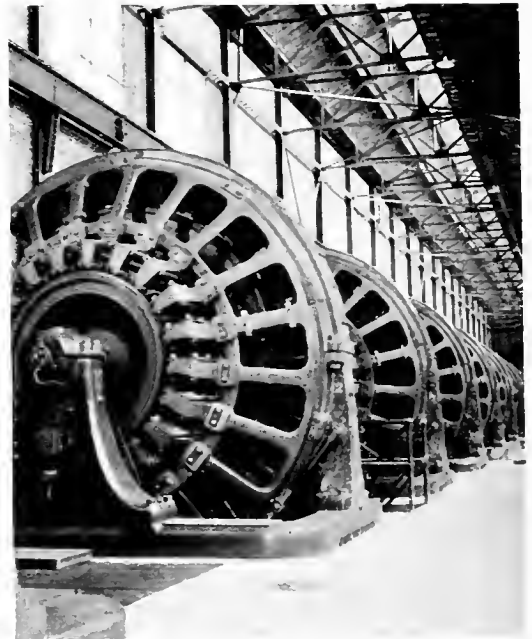
Fig. 4. The Direct-Current Ends of the Converters as installed, showing the moulded asbestos pieces on the brush-holders
