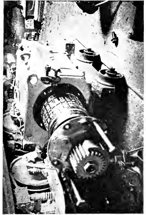
Fig. 14. The armature is supported by jacks which can be readily adjusted to take the weight of the armature off the pole pieces
