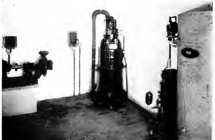
Fig. 8. Shed for the Stationary Vacuum Cleaning Outfit and High Pressure Pumping System in Connection with the "Home Electrical" Exhibit
