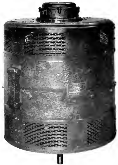
Fig. 19. Main Drainage Pump Motors
