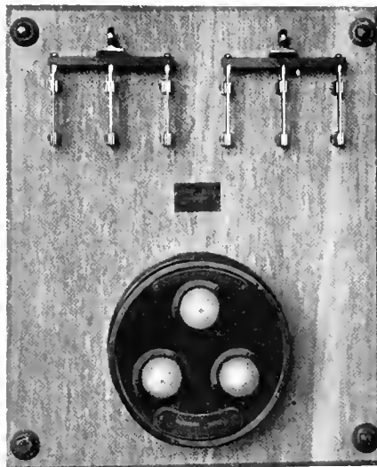
Fig. 21. Electrostatic Synchronism Indicator and disconnecting switches
