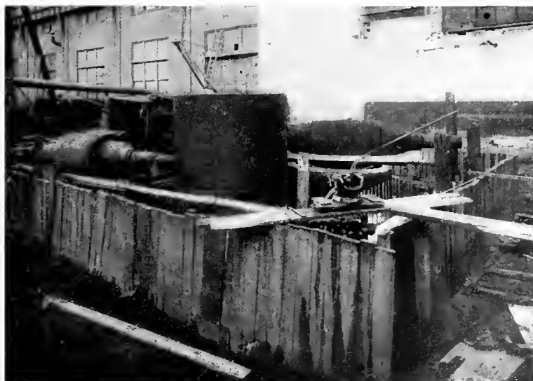
Fig. 2. Loads as placed on the Tank to Facilitate Sinking it into place
