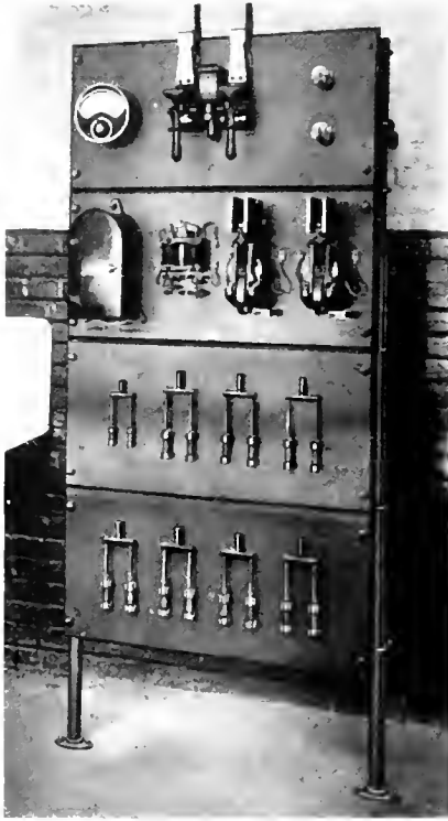
Fig. 10. Switchboard for Controlling the Heating of the Baking Oven
