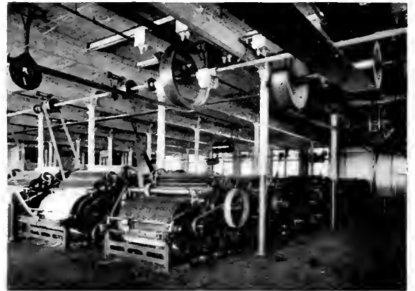
Fig. 7. Typical Group Drive in Card Room
