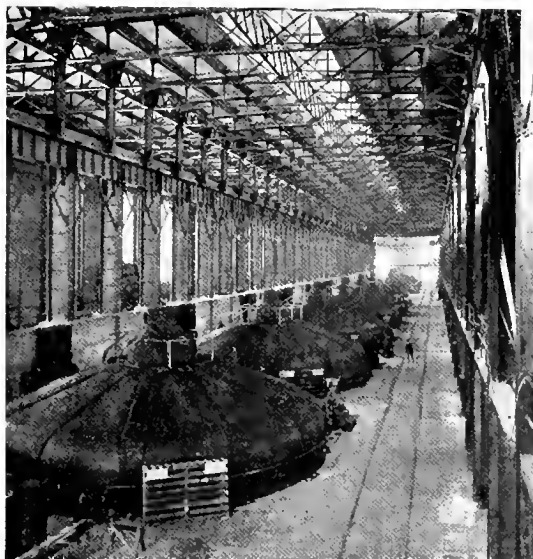
Fig. 5. Interior of Cedars Rapids Power House. Present equipment, nine 10,000 kv-a., 136-pole, 55.6 r.p.m., three-phase, 6600-volt generators. Ultimate equipment, eighteen similar units
