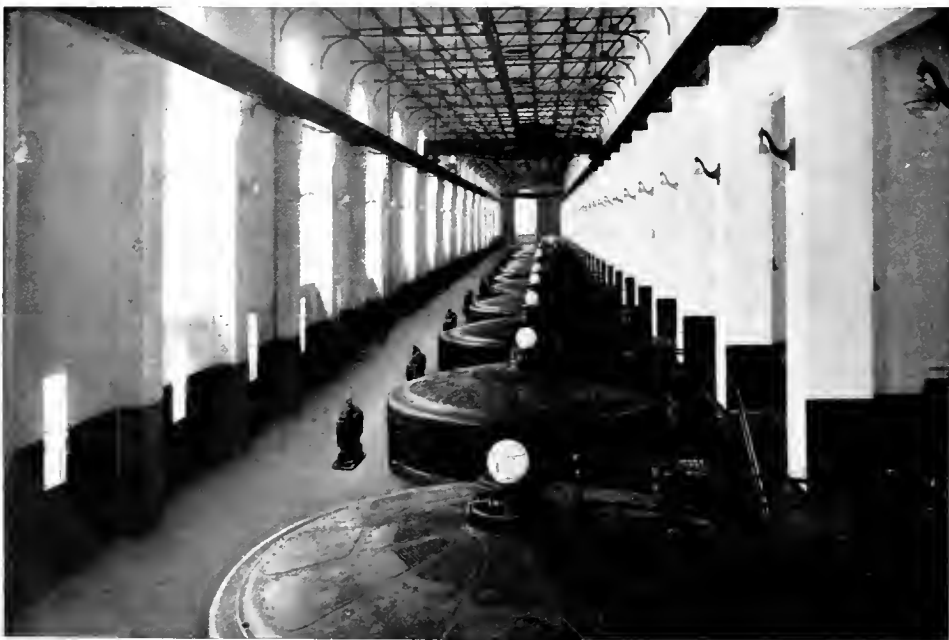
Fig. 3. 9000 Kv-a. Generators, Mississippi River Power Company, Keokuk, Iowa
