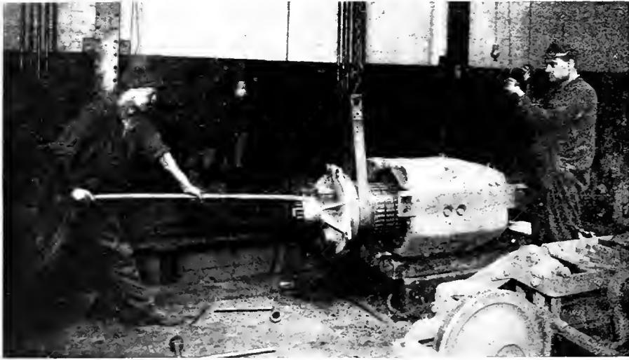
Fig. 4. Removing Armature from a 65-H.P. Box Frame Motor. Lifting strap in position. From the time the motor is off the truck until the armature is on the floor is twenty minutes
