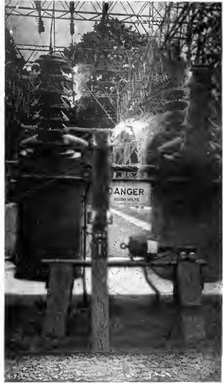
Fig. 6. Telephone Arrester Operating on 118,000 Volts from Power Line
