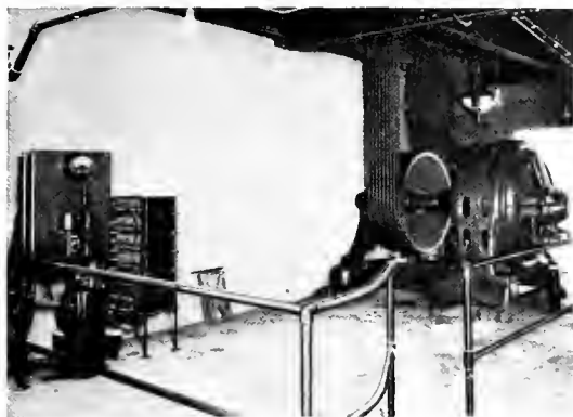
Fig. 19. 200-h.p., Three-phase, 60-cycle, 440-volt, 360-r.p.m., Form P, Three-bearing Motor Driving Bolters and Purifiers in Flour Mill
