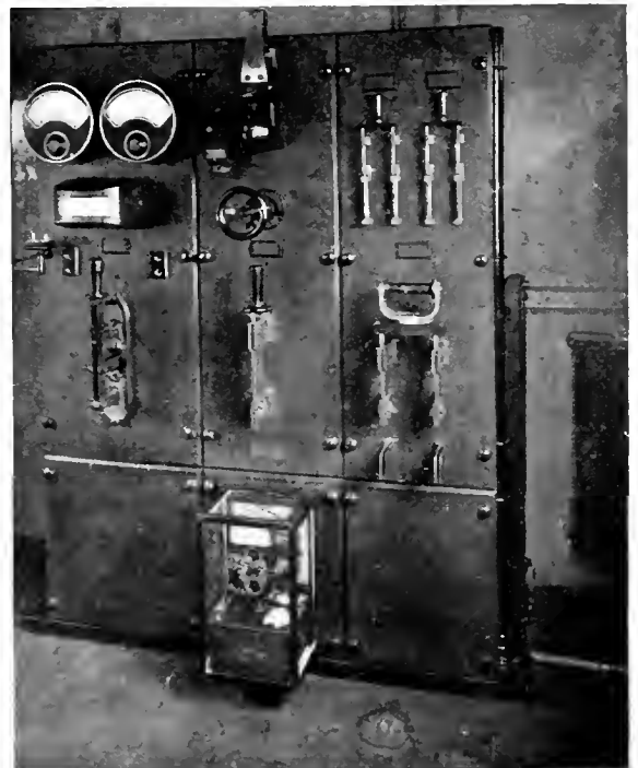
Fig. 3. The Control, Feeder and Starting Panels (left to right) of the Portable Substation Switchboard
