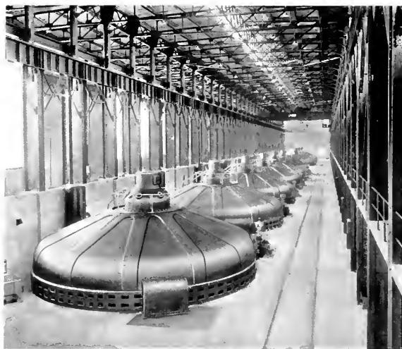
Fig. 10. View of Generator Room
