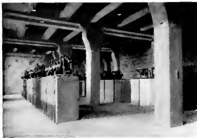
Fig. 18. High Tension Oil Switches, Located on Second Floor of Transformer House
