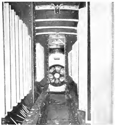
Fig. 21. Center Aisle of Contactor Compartment, Looking Toward Blower, showing Contactor Arc Chutes and Method of Fastening Hatches
