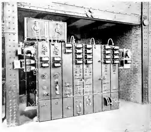
Fig. 6. Main Switchboard in Ingham Mills, New York Power Station, East Creek Electric Light & Power Company
