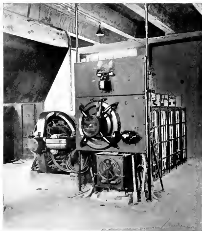
Fig. 13. One Generator Field Rheostat Panel and Exciter
