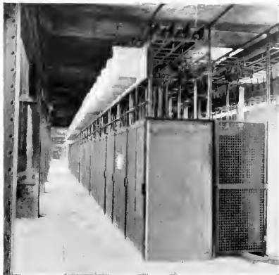
Fig. 19. High Tension Bus Compartment
