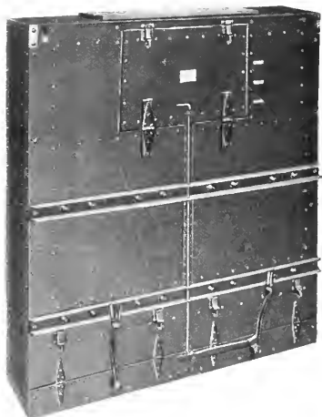
Fig. 2. 3000-volt Switch and Fuse Compartment
