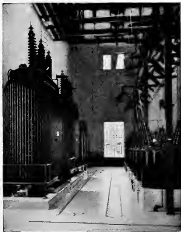
Fig. 19. Chicago, Milwaukee & St. Paul 3000-volt D-c. Electrification Two 2500-kv-a. Three-phase 100,000/2300-volt Transformers and Oil Switches in Moret Substation
