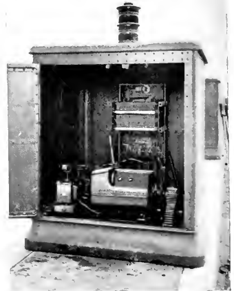
Fig. 28. Rear View of the Control Panel and Cabinet shown in Fig. 27
