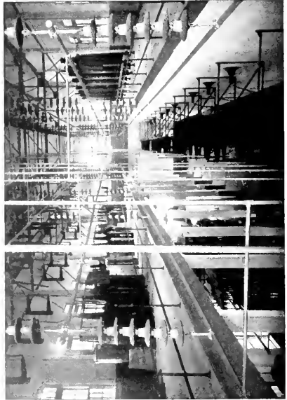
Fig. 16. Butte Substation, Showing 100,000-volt Bus Construction, Great Falls Power Company
