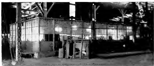
Fig. 19. Motor House in the Plant of the American Iron and Steel Company Containing the Motor and Control for 8-inch Roughing and 10-inch Finishing Frames
