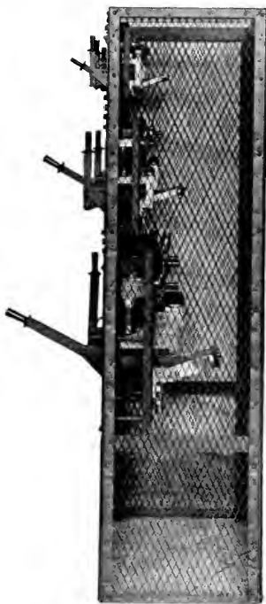
Fig. 4. Safety First Switch Panel Side View
