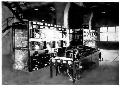
Fig. 17. Control Desk and Instrument Board in Transformer House for Transformers on Outgoing Lines; and in background, Auxiliary Board for Battery, Lighting, Heating, etc.
