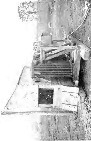
Fig. 9. Out door type of Portable Transformer Station for the Excavator shown in Fig. 8
