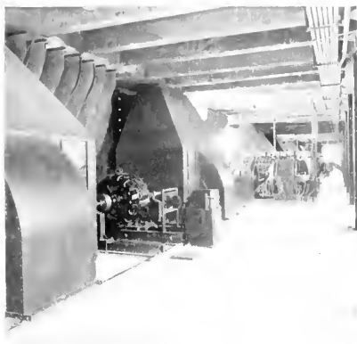
Fig. 15. Motor Operated Fans for Generator Ventilation
