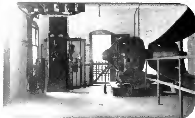
Fig. 31. 250-h.p. Induction Motor Belted to Mine Fan
