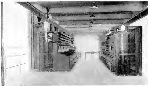
Fig. 16. Main Control and Instrument Switchboard
