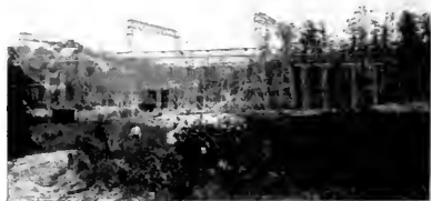
Fig. 5. A General View of the Jackson Shoals Substation
