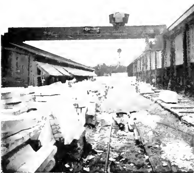
Fig. 6. 30-ton Crane Operated by A C Motors
