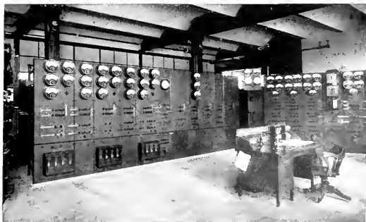
Fig. 11. Main Switchboard, Volta Plant, Montana Power Co. Great Falls, Montana
