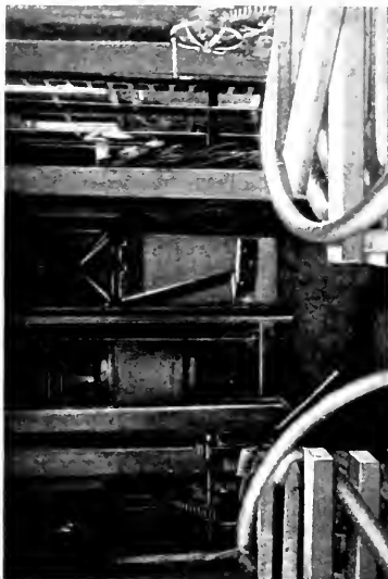
Fig. 13. Landing Floor of Three Compartment Penrose Shaft. Two Thousand Gallon per Minute Sinking Pump working in the right-hand compartment, Companion Pump about to be lowered in the left-hand compartment. Hoisting Cage in center. Coiled Electric Power Cables for Pump Motors shown in right and left foreground
