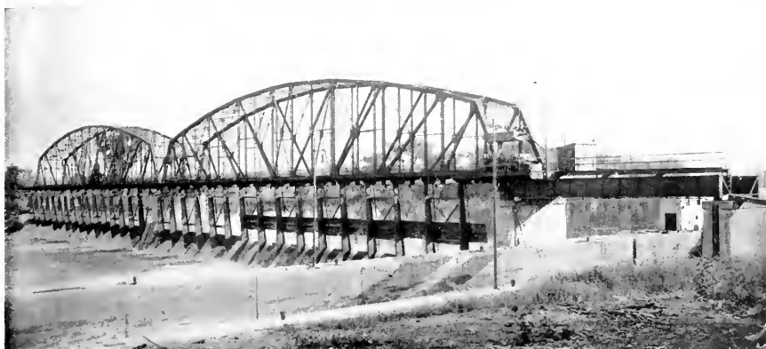
Fig. 12. Movable Dam across Mohawk River, of which type there are eight between Scotia, N. Y., and Fort Plain, N. Y., varying in length from 370 to 590 ft. and raising the river level 14 ft. at Lock 8; 15 ft. at Locks 9 and 10; 12 ft. at Lock 11; 11 ft. at Lock 12, and 8 ft. at Locks 13, 14 and 15
