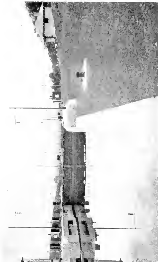
Fig. 25. Typical View of Lock Receiving Power from Adjacent Lock. The sheet iron cabinets shown in the wall enclose the gate valve, capstan motor, and control panels
