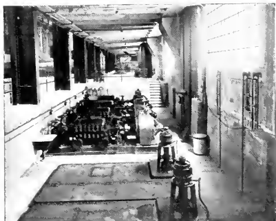
Fig. 9. Pump Pit Containing Governor Pumps and Oil Pumps
