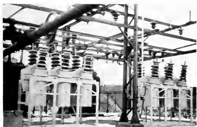
Fig. 8. Outdoor Oil Break Circuit Breakers
