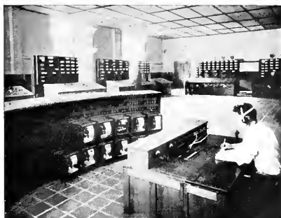
Fig. 9. Control Switchboard, Mississippi River Power Company, Keokuk, Iowa
