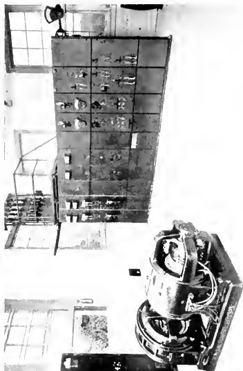
Fig. 18. Typical Substations: 35-kw., 1200-r.p.m., motor-generator set and switchboard. Induction motor 50-h.p., 1200-r.p.m., 2200-volt, three phase, 40 cycle; generator 35-kw., 1200-r.p.m., 250-volt, compound-wound, commutating-pole
