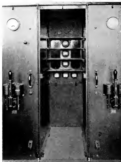
Fig. 11. Safety First Truck Type Switchboard, One Truck Removed to Show Rear of Compartment
