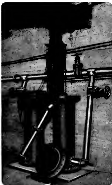
Fig. 12. Electric Air Heater for Hoist
