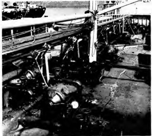
Fig. 4. Arrangement of Motor Drive for Cargo Pumps on S. S. La Brea
