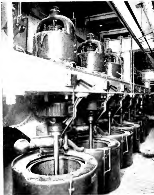
Fig. 10. Motor Built in Sugar Centrifugals. Individual Drive for sugar centrifugals is usually accomplished by horizontal motor and quarter turn belt for each centrifugal
