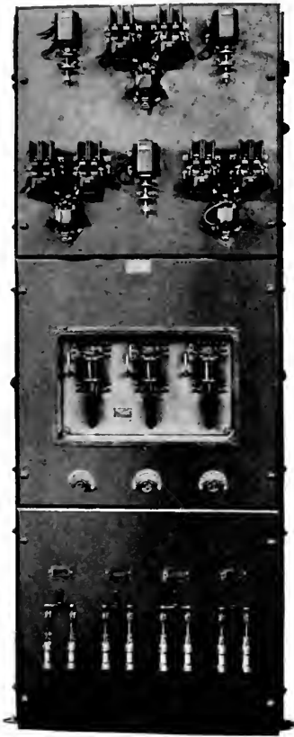
Fig. 17. Automatic Electrode Regulating Panel for Control of Arc Furnaces
