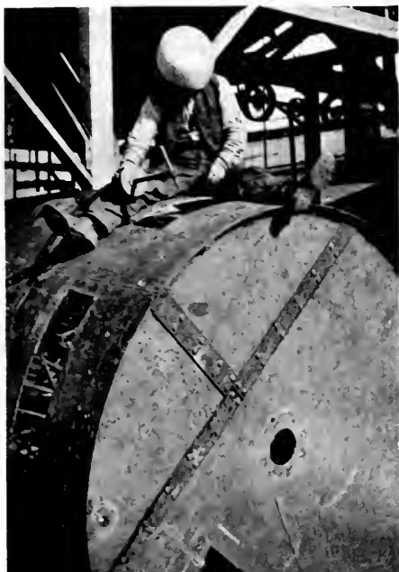
Shell for Steel Furnace showing tuyere openings and bolt holes cut by arc. The position of a new electrode in the holder is clearly shown
