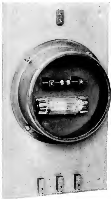
Fig. 9. Spark Tube Panel for Spark-tube Discharge Alarm
