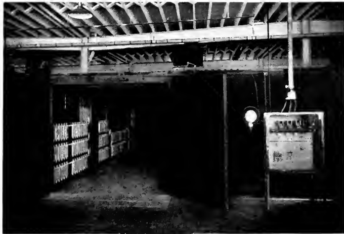
Fig. 37. Electrically Heated Japanning Oven in Automobile Manufacturing Plant
