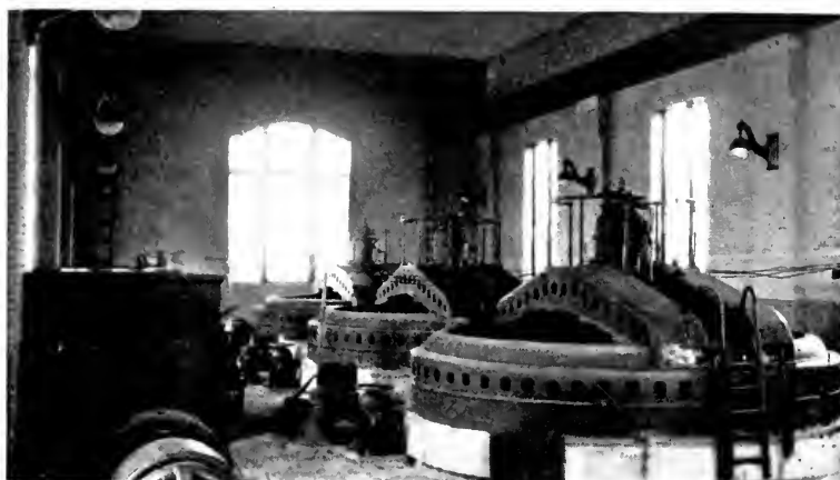
Fig. 8. General View of the Interior of the Automatic Generating Station. A Motor-driven Exciter is shown in the Lower Left-hand Corner
