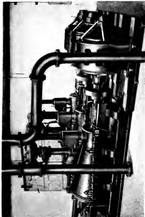
Fig. 14. Three 150-h.p. Induction Motors Driving Jordans. Kimberly-Clark Company, Kimberly, Wis.
