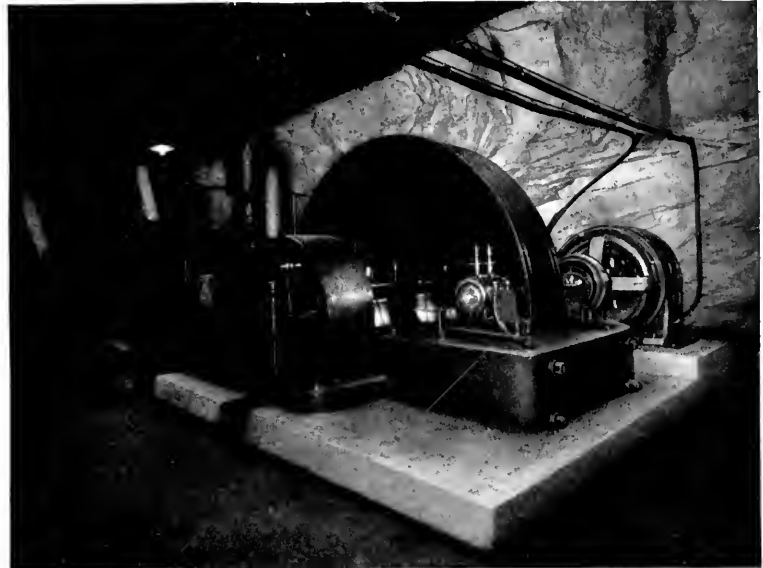
Fig. 6. Crank end of 1500-gallon Duplex Double-acting Prescott Station Pump showing enclosed Herring Bone Gear, Flexible Coupling and 300-h.p. Wound Rotor Induction Motor. Fossil Slope No. 8
