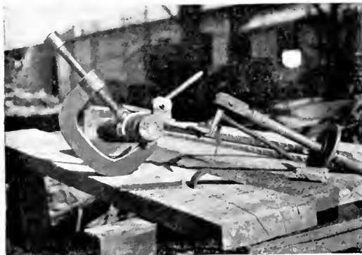
Clamps and Copper Bars for Connection to Work. Electrode Holder with Carbon Electrode almost Consumed
