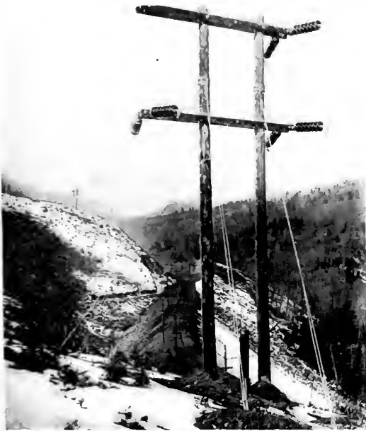
Fig. 3. 100,000-Volt Transmission Tower for Long Span
