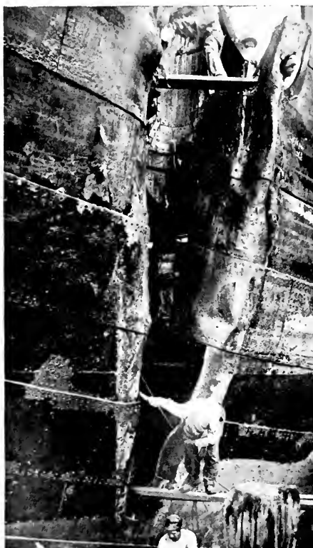
Fig. 1. Hole in Side of Steamship Caused by Collision. Arc Welding Set Used in Making Repairs
