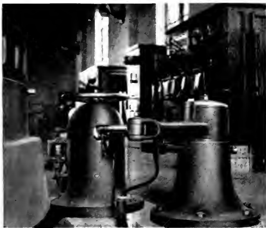
Fig. 7. Waterwheel Gate Control in the Foreground and Automatic Control Cabinet Panels in the Background
