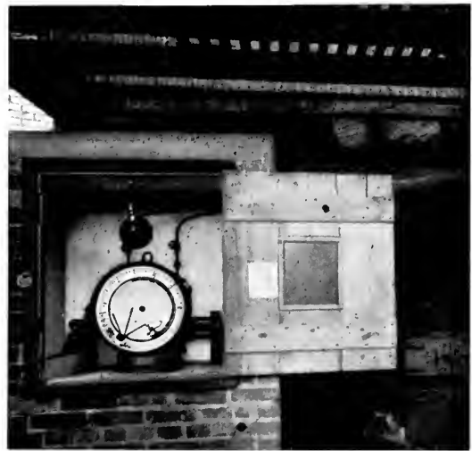
Fig. 4. Indicating Recording Integrating Flowmeter installed in a 14-inch line supplying steam to the mills of the Pennsylvania Steel Company, Steelton, Pa.
