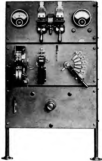
Fig. 20. Arc Welding and Generator Control Panel
