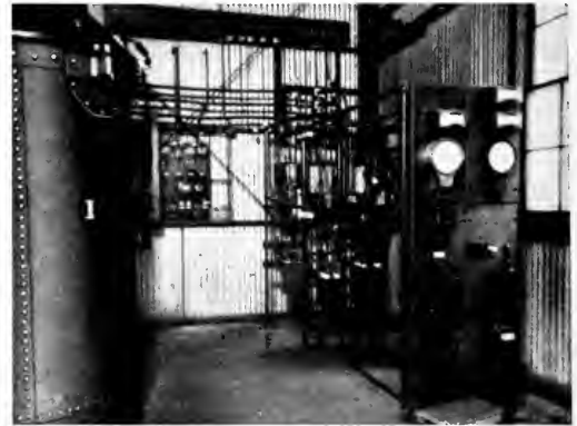
Fig. 3. Feeder Switches and Transformer Room
