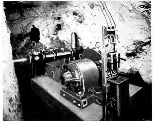
Fig. 5. Typical Bottom Pump Installation showing 5 by 7 Aldrich Triplex Pump Driven by Fully Enclosed 15-h.p. Squirrel-cage Induction Motor through Flexible Coupling
