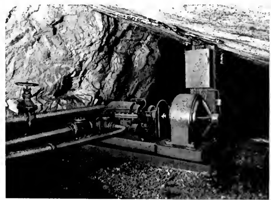
Fig. 8. 400-gallon 4-stage Centrifugal Pump, Driven by 100-h.p. Squirrel-cage Induction Motor for Furnishing Domestic Water Supply. Muscada Slope No. 4
