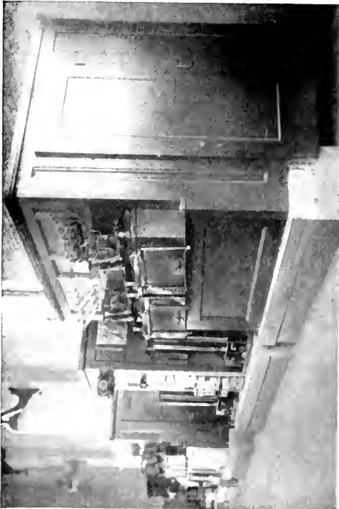
Fig. 3. Panel Cabinets and Automatic Equipment for Control of the Generating Units
