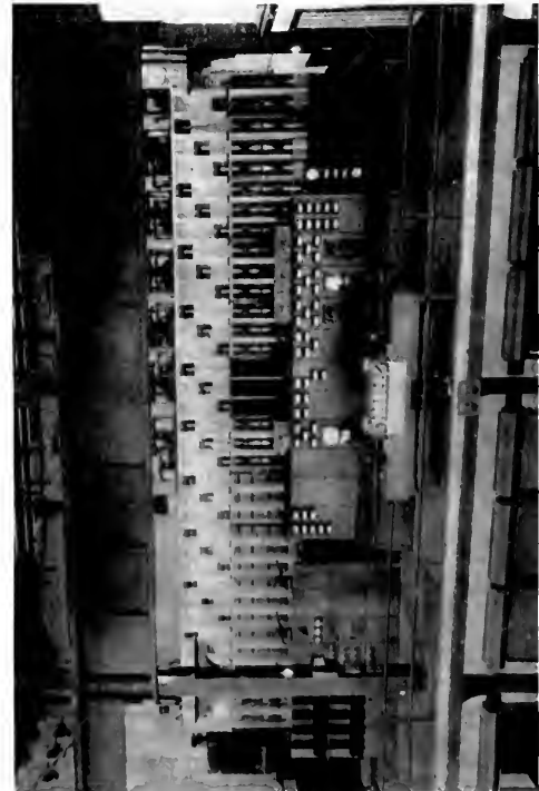
Fig. 9. View of Switchboard Operating Gallery
