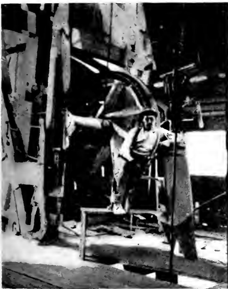
Fig. 5. Drilling a 1900-ft. oil well by electric power with standard cable tools in the Midway field in California
