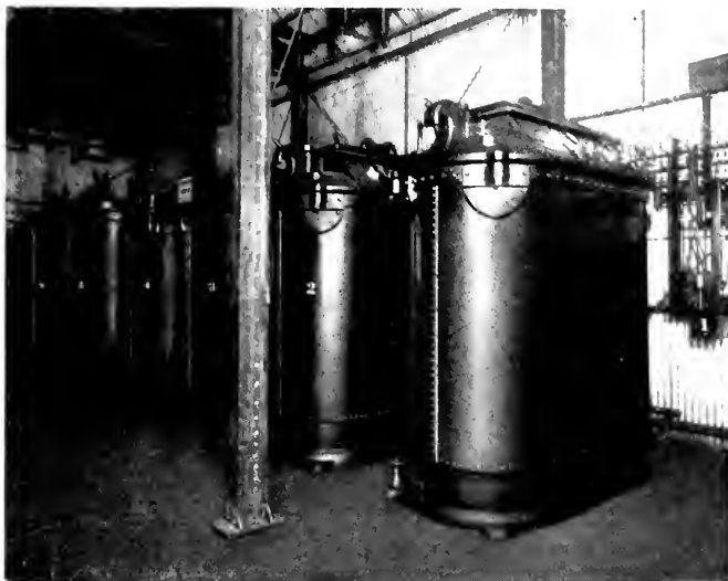
Fig. 4. View in Substation of Bunker Hill & Sullivan Company Showing Seven 650 kv-a. 60,000/2300-volt Transformers
