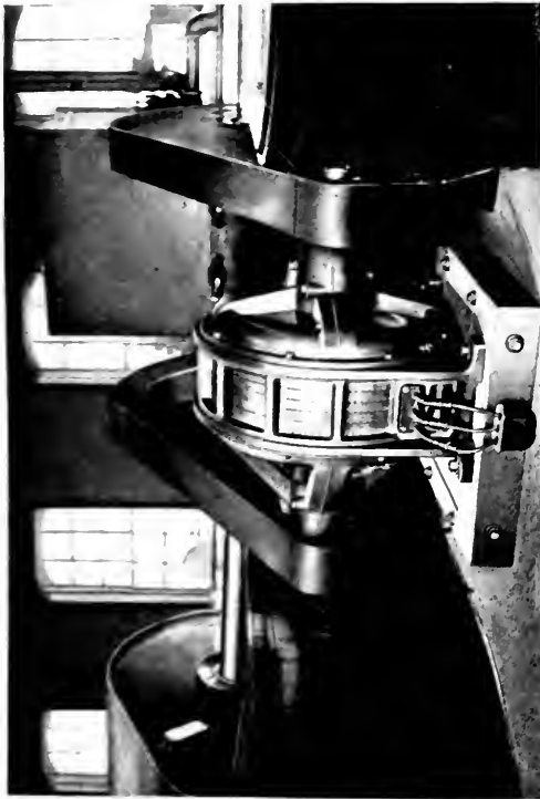
Fig. 7. 150-h.p. Induction Motor Driving Two Beaters through Chain Belts. Kimberly-Clark Company, Kimberly, Wis.
