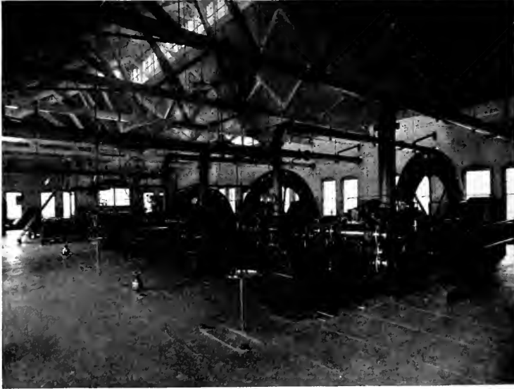
Fig. 4. Two Synchronous Motor-driven, Twin, Two-stage Air Compressors with Former Steam Ends Removed
