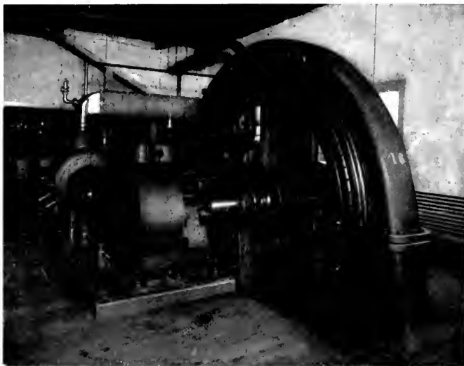
Fig. 20. 2400 Cubic Foot Ingersoll-Rand Air Compressor Driven by 400-h.p., 2200-volt Induction Motor
