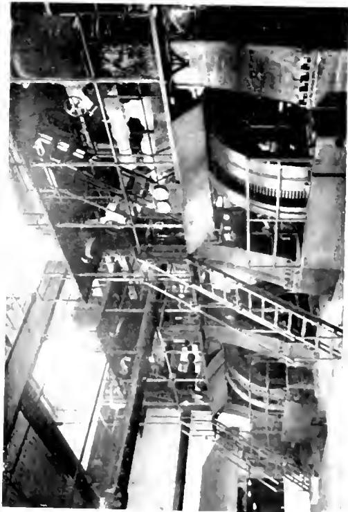
Fig. 12. 1,000-ton Refrigerating Machines Driven by Two 500 kv. a., 6,000 volt Synchronous Motors
