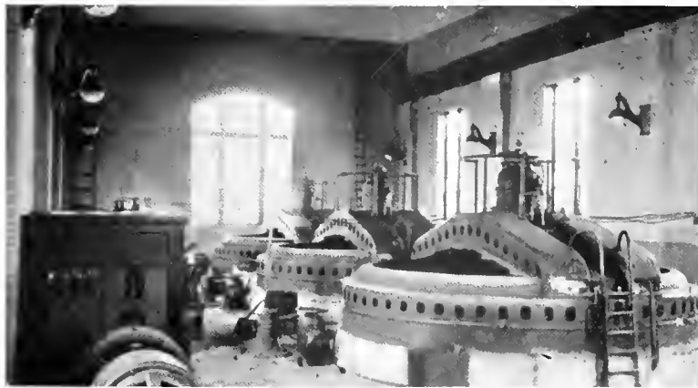
Fig. 23. Automatic Hydro-electric Generating Station, Iowa Railway & Light Company. General view showing three 60-cycle, 500 kv-a., 60-r.p.m., 2200-volt automatically-controlled generators
