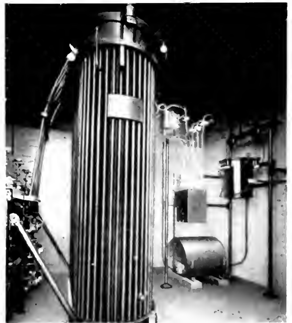
Fig 5. Near View of 240 kv a Starting Transformer, Motor Operated Oil Breaker and 5 kw Control Transformer
