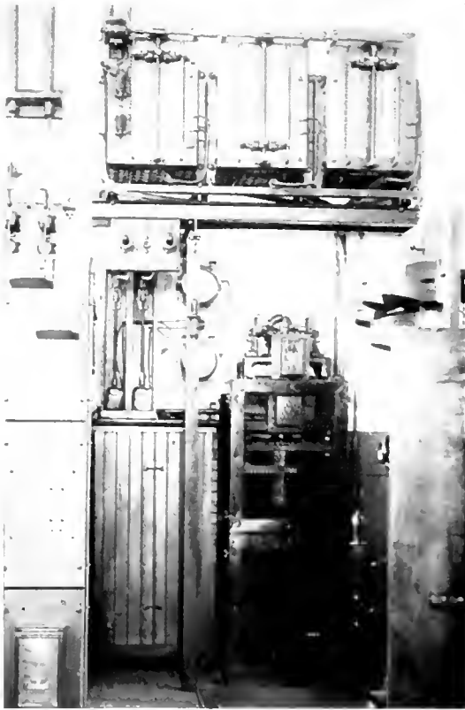
Fig. 12. Complete Motor Operated Contact Making Wattmeter Unit and Motor Operated Generator Voltage Lowering Rheostats Located Above the Wattmeter in the Janney Substation
