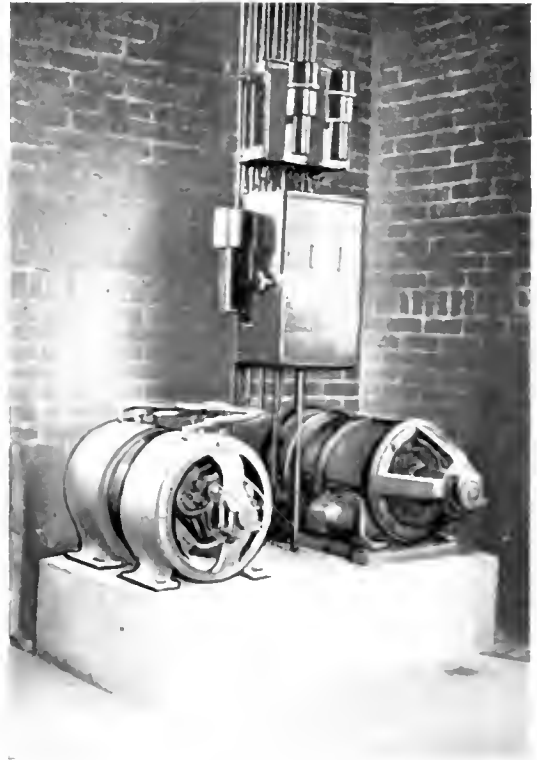
Fig. 6. Battery Charging Motor-generator Set and Alternating-current Emergency Motor-generator Set in a Signaling Substation, Philadelphia & Reading Railroad
