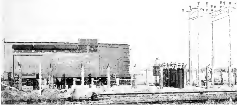
Fig. 6. The Automatic Railway Substation and Its Outdoor Transformer Installation
