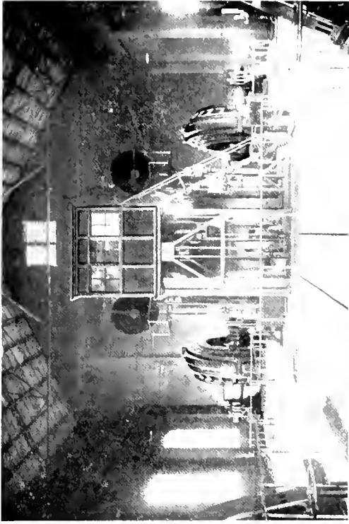
Fig. 2. General View of the Electrically Driven Hoist, New Modderfontein Gold Mine
