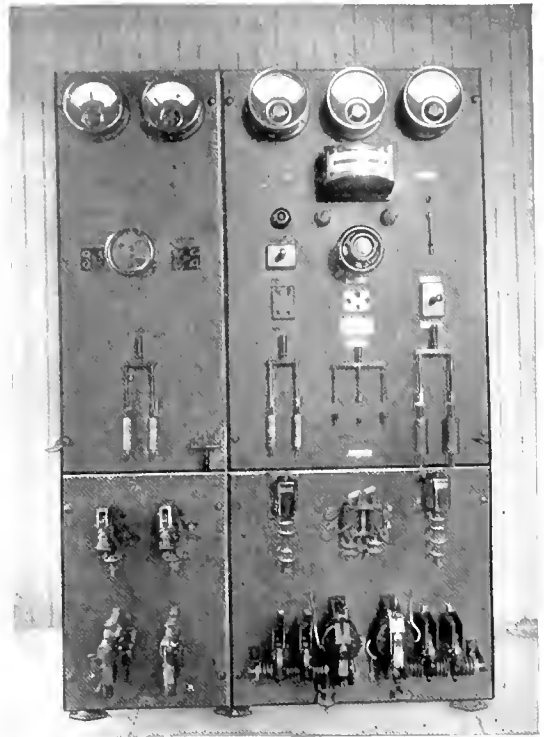
Fig. 3. Switchboard, Boston Switch-Central Falls Signal Tower, New York, New Haven & Hartford Railroad, Pawtucket, R. I.
