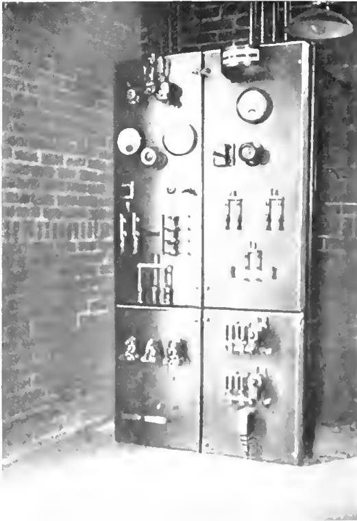
Fig. 5. Switchboard in a Signaling Substation, Philadelphia & Reading Railroad
