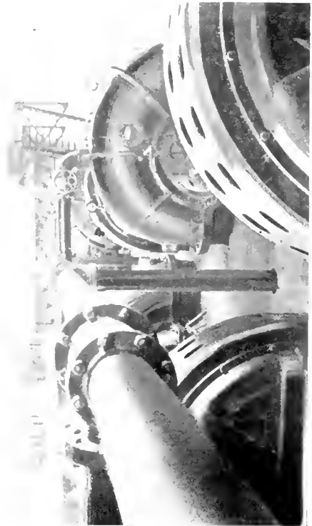
Fig. 3. A Partial View of the Main Motor-driven Pumps, Six in Number, Each Having a Capacity of 175 Second Feet of Water
