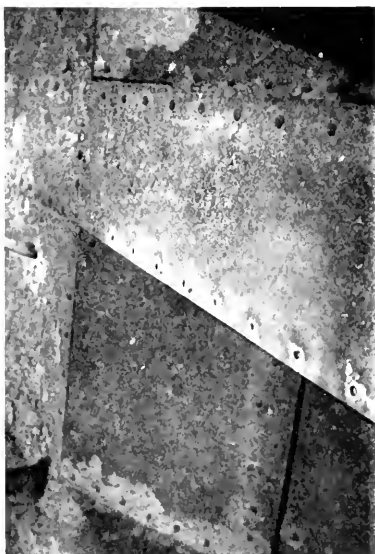
Fig. 3. Sample of floor work. These eight rivets were burned at the rate of 400 per hour
