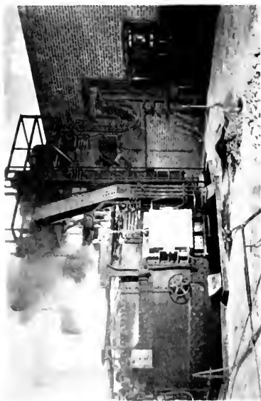
Fig. 21. 40-ton Furnace Showing Control Panels on Right and Electric Motors on Platform Above
