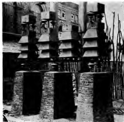
Fig. 3. 37,000-volt, 3-phase, Outdoor Type Oxide Film Lightning Arrester, Chee Hsin Cement Company, Ltd., Tongshan, North China
