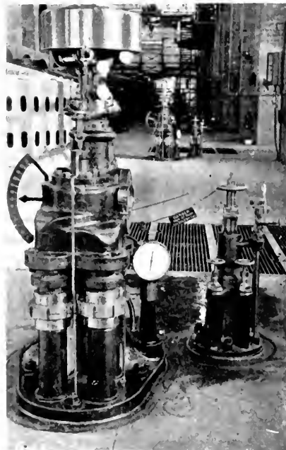
Fig. 8. A Hold-off Sign, Chain, and Lock which prevent the operation of either the governor or the hand controls. The turbine gates are half-way open to prevent the formation of an accumulation of headgate leakage that might move the rotating element
