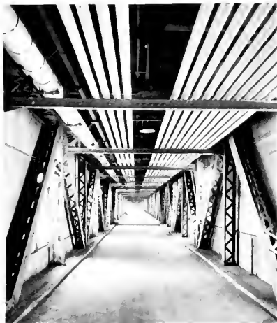
Fig. 10. Arrangement of 14 Feeder Lines Carried on Roof Beams of Covered Bridge from the Power Station to Mill No. 8
