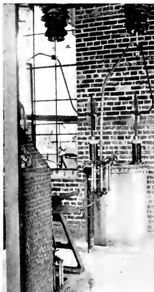
Fig. 3. Precipitator Transformer and Synchronous motor-driven Mechanical Rectifier
