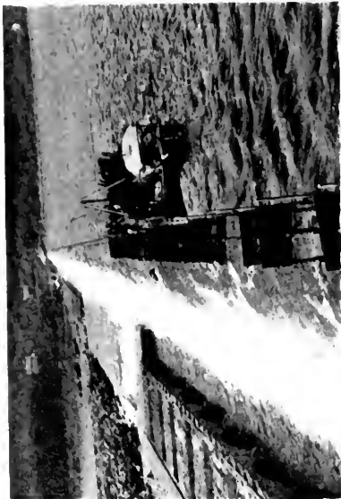
Fig. 2. Use of Guard Pins for the Security of Floating Equipment on Flashboard Work. Anchors are also used for the purpose.
