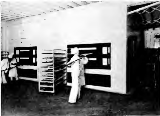
Fig. 14. A Typical Installation of Electric Brick Ovens. This bank has a total capacity of approximately 1200 one-pound loaves per hour
