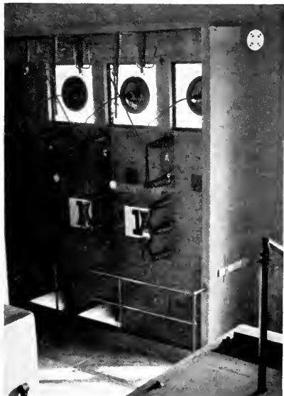
Fig. 3. Sleet Prevention Facilities at Receiving Station. The upper disconnectors serve to short circuit the transmission line when heating current is to be circulated. The disc in the upper right-hand corner carries eight 8-volt lamps in parallel connected to a series transformer in the short-circuiting connections and indicates when the heating current is on.
