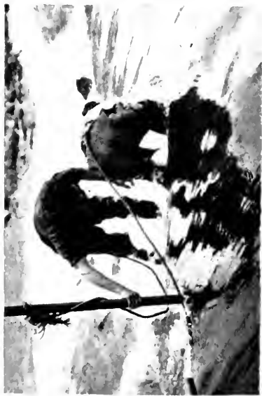
Fig. 3. When men must get out on the crest of a dam, handlines about the waist are necessary.
