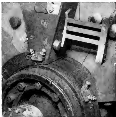
Fig. 6. Barrier Removed for Inspection After 50 Maximum Short Circuits as Shown in Fig. 5
