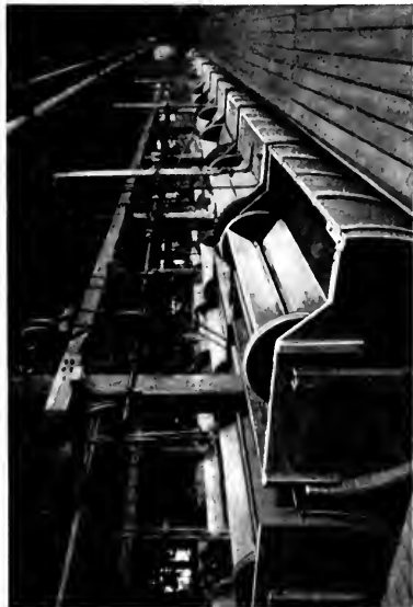
Fig. 8. View of a lime yard in which there are 164 lime reels group-driven by twelve 7½-h.p. motors. John R. Evans Co.
