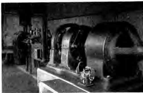
Fig. 5. Motor-generator Set and Control (225-h.p. induction motor; 150-kw., 75-volt generator) for supplying energy to five operators per shift
