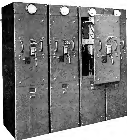
Solely Enclosed Standard Unit Switchboard made up of Type FK- 20 Oil Circuit Breakers as Draw- outs
