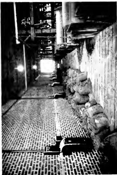
Fig. 9. End view of the lime yard showing the location of the hand-starting compensators, reversing switches, and safety switches controlling the motors that drive the lime reels
