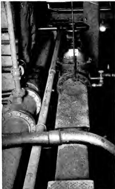
Fig. 9. The hazard of reaching valves difficult of access can in many cases be lessened by the use of non-slip tread plates on the piping
