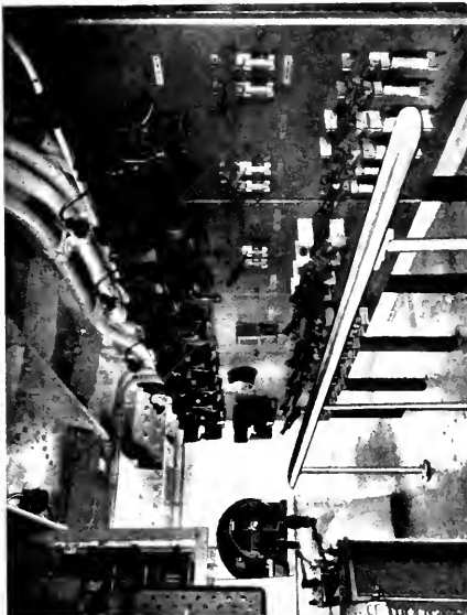
Fig. 5. Pump Control Room Showing Auxiliary Distribution and Control Board for Cargo Oil Pumps. Pump motor controllers, resistance grids, and ventilating motor at the left
