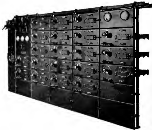
Fig. 6. Twenty-circuit Battery Charging Switchboard for Constant-current or Series-resistance Charging
