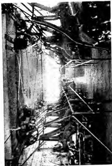
Fig. 5 One 5-h.p. and One 7 1/2-h.p. Induction Motor Driving Five and Six Glazing Jacks, Respectively
