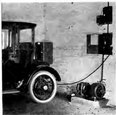
Fig. 4. Taper or Modified Constant-potential Charging Motor-generator Set in Home Garage
