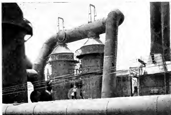
Fig. 7. Two Precipitator Units Handling Blast Furnace Gases
