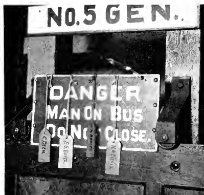
Fig. 10. An Application of Hold-off Signs to prevent mistakes. The generator disconnecting switches cannot be closed without moving the door, and the door cannot be moved until the sign is removed. Workmen's tags, placed and removed by the men who are reported on, decrease the likelihood of the sign being removed until each of the workmen has reported clear.
