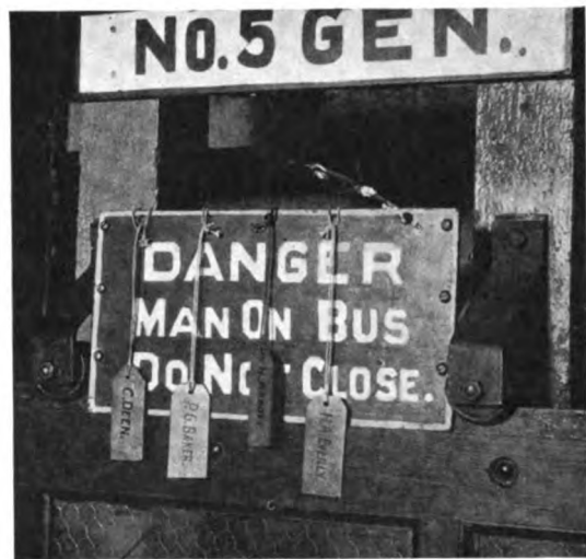
Fig. 10. An Application of Hold-off Signs to prevent mistakes. The generator disconnecting switches cannot be closed without moving the door, and the door cannot be moved until the sign is removed. Workmen's tags, placed and removed by the men who are reported on, decrease the likelihood of the sign being removed until each of the workmen has reported clear.
