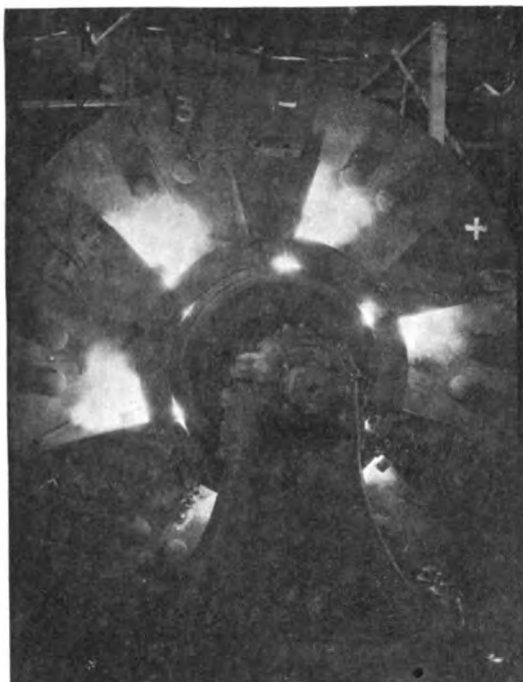
Fig. 3. End View of Flashing Caused by Short Circuit Recorded in Fig. 1. Machine equipped with radial brush-holders and barriers
