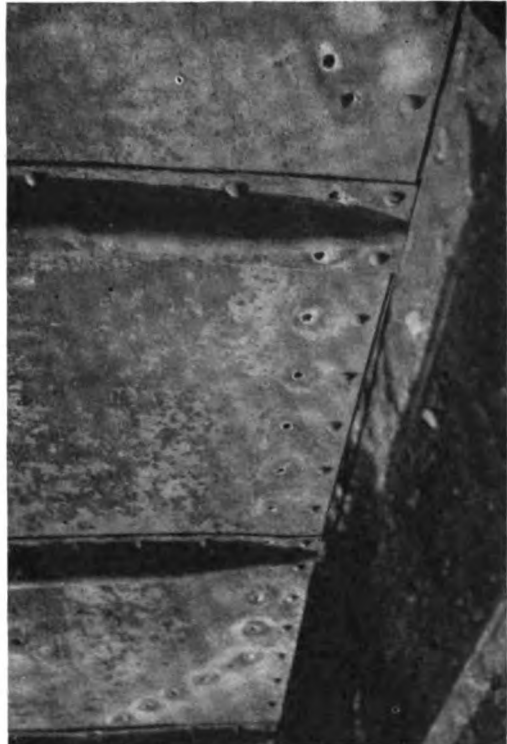
Fig. 4. After the Rivets are Backed. The rivet holes are not damaged by the arc
