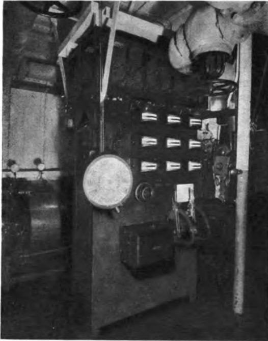
Fig. 2. The Maneuvering Platform of an Electrically Driven Vessel. The ship is held under perfect control by the two small levers near the bottom of the panel
