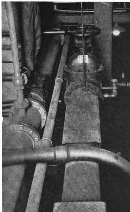
Fig. 9. The hazard of reaching valves difficult of access can in many cases be lessened by the use of non-slip tread plates on the piping
