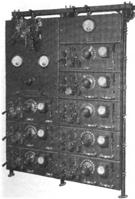
Fig. 8. Eight-circuit Battery Charging Switchboard for Constant-current or Series-resistance Charging with Automatic Cut Off and Ampere-hour Meters in Each Circuit
