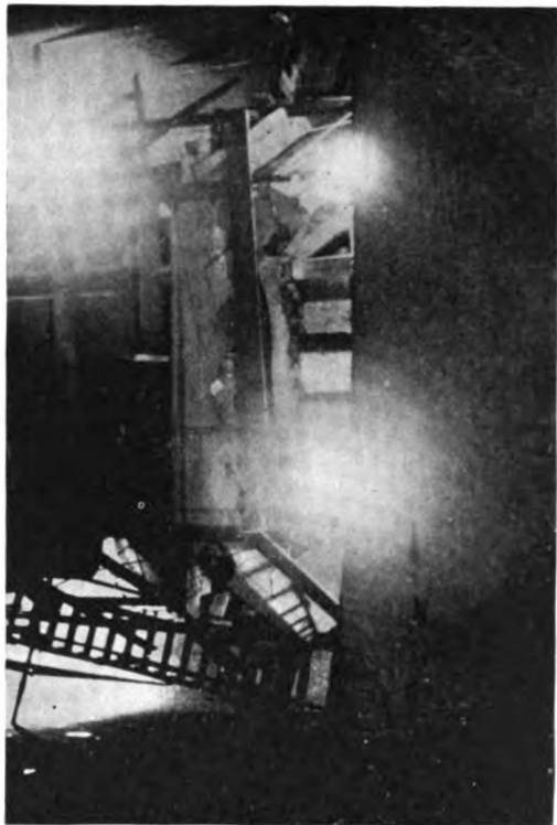
Fig. 4. The use of a stairway instead of a ladder in the scaffolding for this wheel-pit job not only made the work safer but expedited it
