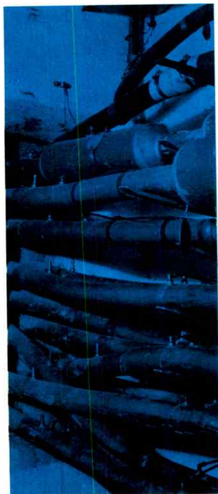
Figure 4. Photo shows crowded cable ducts.
