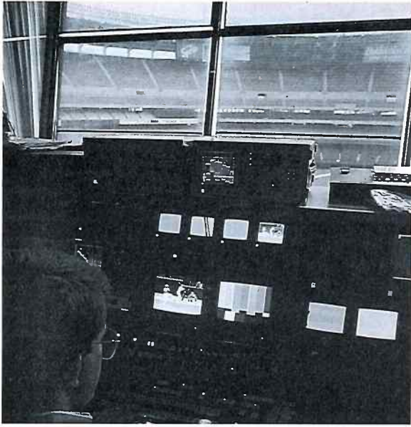
Fig. 4: The control room at Riverfront must be operating perfectly on gameday, certainly a challenge considering the miles of cables and network feeds.
