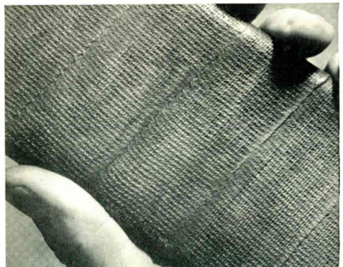
Fig. 3—After ten years' service the Aquadag-treated slot portion of this coil from a 13.8-kv generator showed no deterioration.
