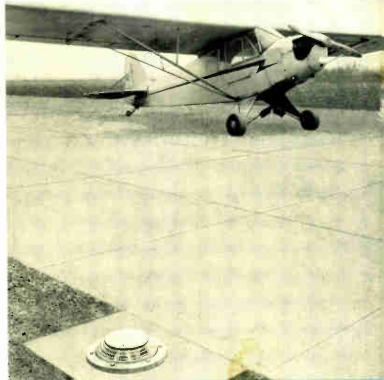
These lights, buried along airport runways to mark the runway boundaries, must be unobtrusive physically but prominent optically. Though small, their inherent strength must be great should a plane strike them.
