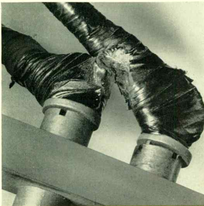
Fig. 3—This lead-to-lead fault developed on the full-wave impulse. Fusion of the copper resulted from power follow.
