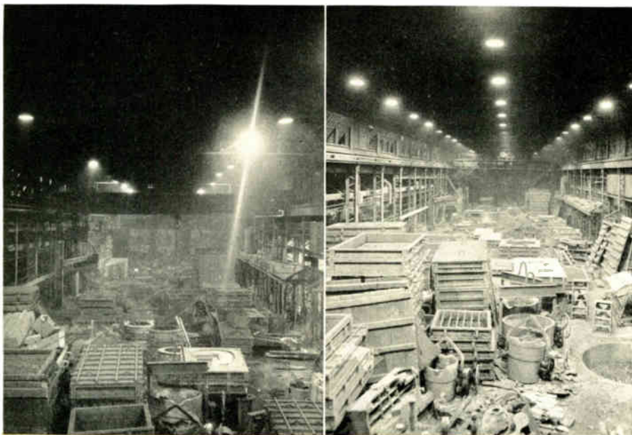
The difference in illumination in large areas between an ordinary lighting system and a properly engineered Millite installation is shown by before and after views.
