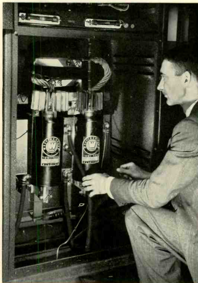
This pair of ignitrons is mounted in a cabinet for resistance-welding control. They each furnish 200 amperes at 440 volts for controlled periods of between two and thirty cycles.
