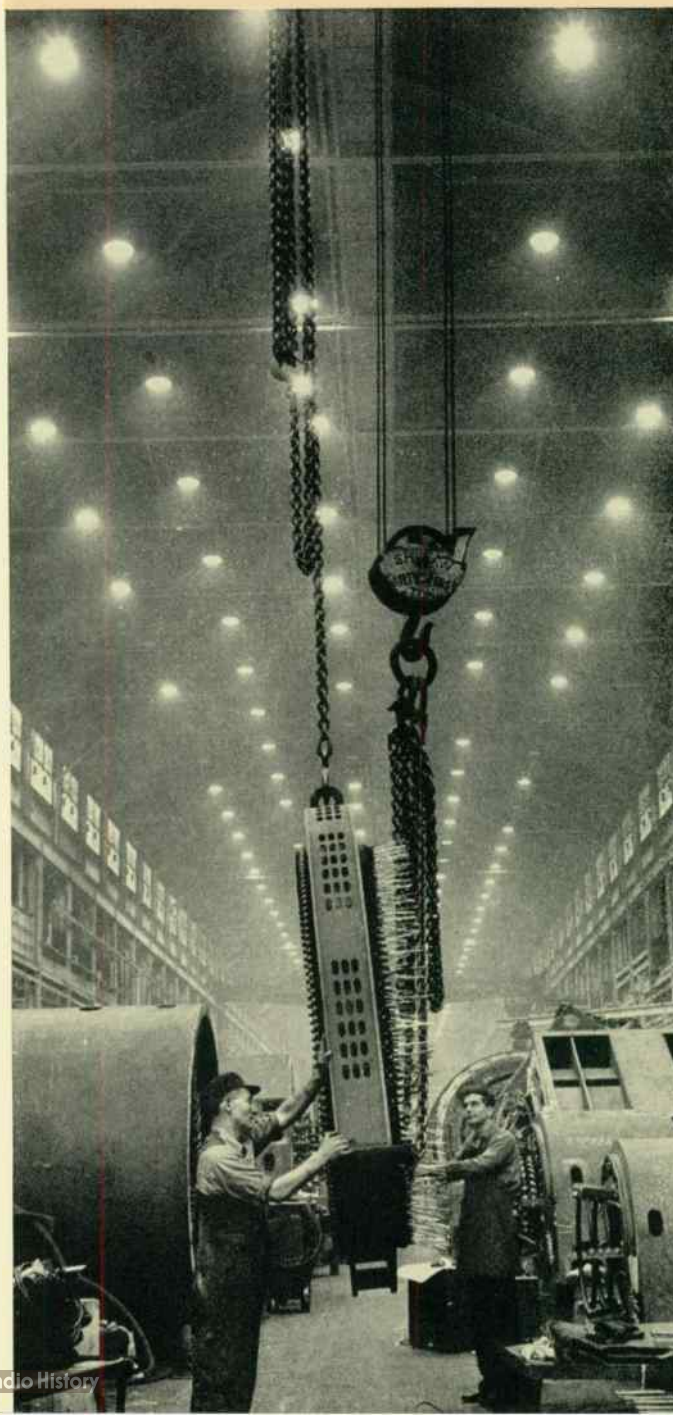
This high bay installation of 1000-watt A-H12 lamps provides high-level, low-maintenance illumination for general shop purposes, material handling, and accurate machining.
