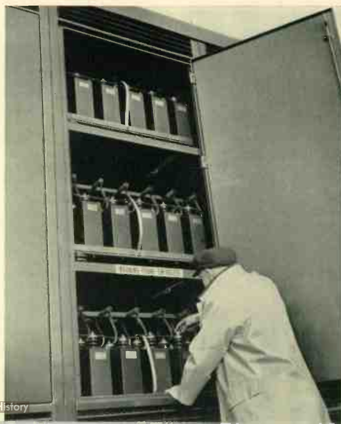
Capacitor units in the 10 000-kvar bank.
