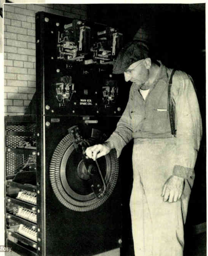
Fig. 9—The motor-operated rheostat controlled by the exciter-rheostatic regulator element is placed in a small cubicle. The contactor panel is located in the upper corner.
