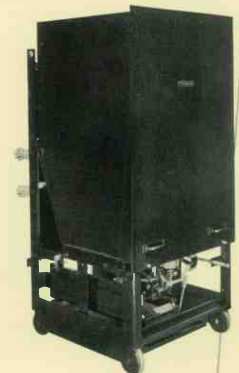
A typical five-kv, removable, magnetic air breaker. The right-hand face of the barrier assembly is steel for protection to operating personnel. When the breaker is in the disconnected position, removal of the barrier exposes the arc chutes and contacts for periodic inspection and maintenance.
