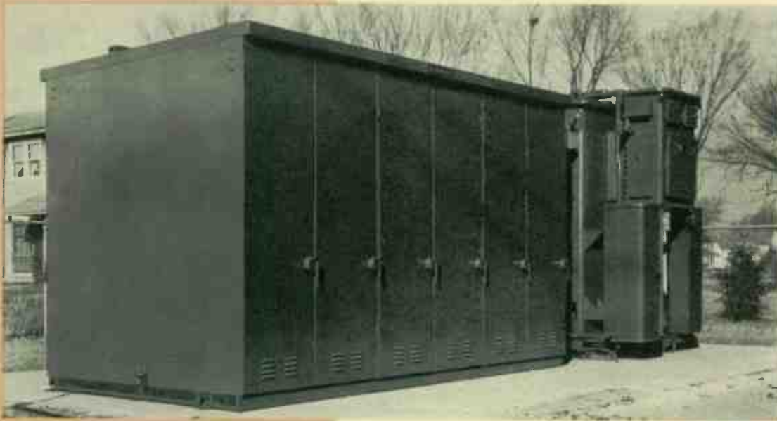
A unit-substation installation. Switchgear at the left controls breaker for four network feeders. The transformer at the right has tap-changing control to maintain voltage. The use of underground sub-transmission supply prevents exposure of live parts, thus safeguarding the residents of the neighborhood as well as the costly electrical apparatus.
