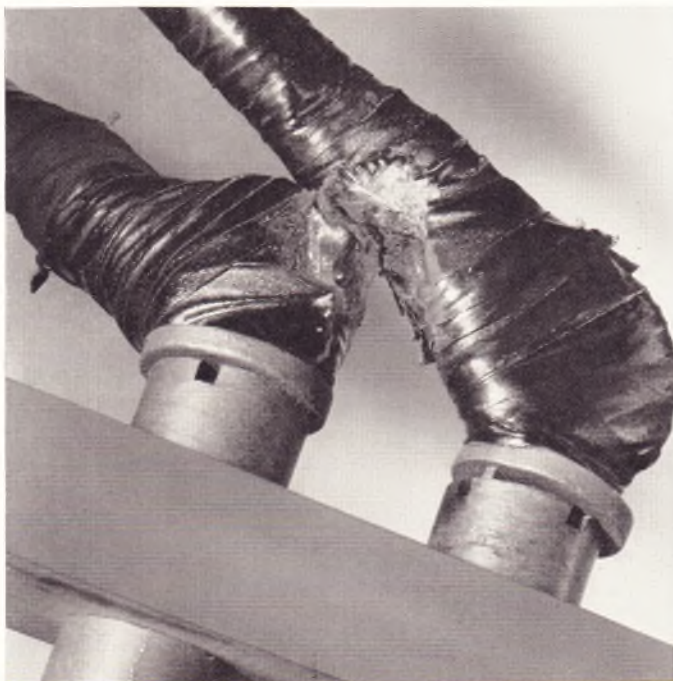
Fig. 3—This lead-to-lead fault developed on the full-wave impulse. Fusion of the copper resulted from power follow.
