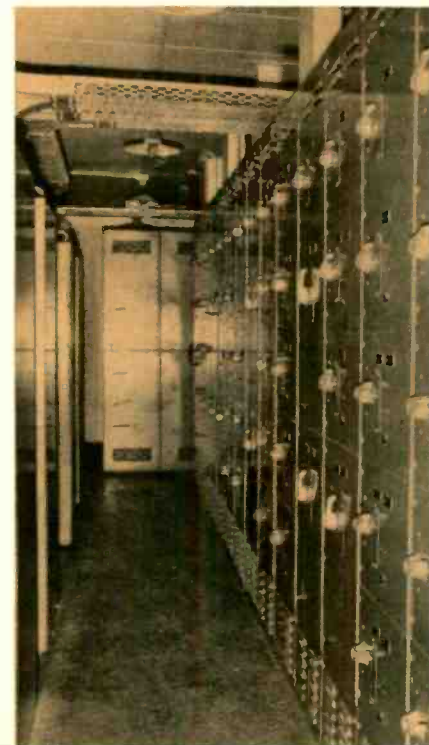
Control center in a refinery.
