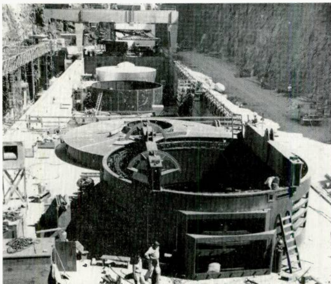
At the Idaho Power Company's Hells Canyon development on the Snake River, three of the four 100 111-kva waterwheel generators at Brownlee Dam are shown during construction.
