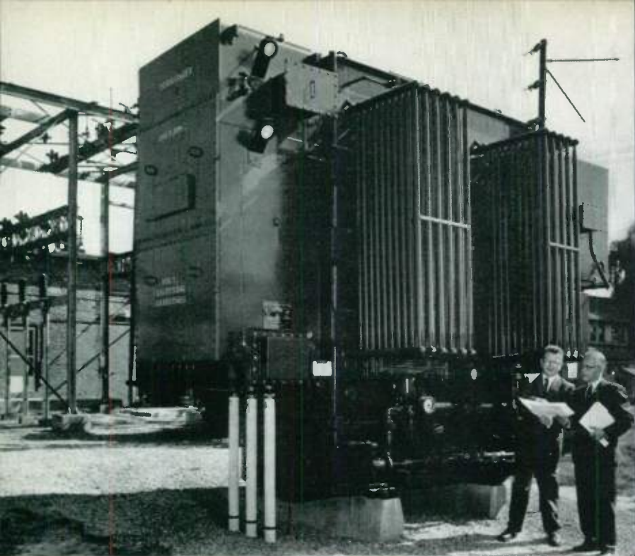
Fig. 4—The exterior of 7500-kva unit.
