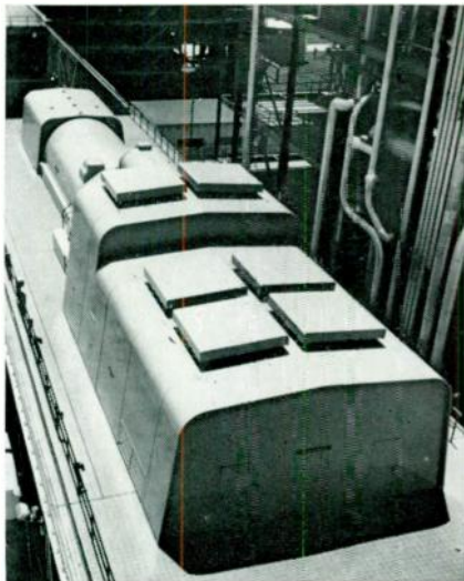
This 352-mva turbine generator unit went into commercial operation at the Houston Lighting & Power Company's W. A. Parish plant in March 1961. Steam conditions for the tandem compound turbine are 2000 psig, 1000 degrees F, with re-heat to 1000 degrees F. The generator is inner cooled, and its 352-mva design rating corresponds to 45 psig hydrogen gas pressure.
