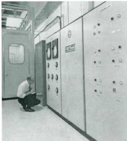
Gauges indicating pressures, pressure differentials, temperatures and humidity are mounted on the control panel, along with operating controls for the air conditioning system, the communications system, and equipment to regulate the environment.
