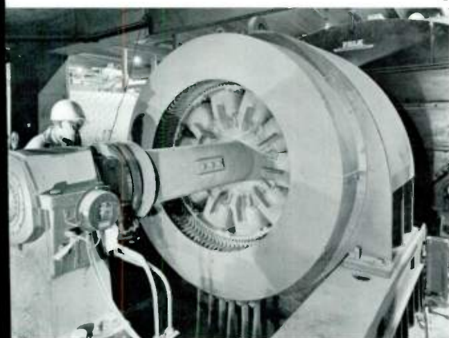
4) LARGE ROD AND BALL MILL used for raw grinding at the Marquette plant is driven by this 3000-horsepower synchronous motor. In the background is one of the plant's smaller ball mills for finish grinding.
