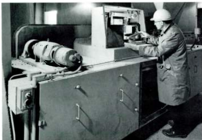
1) BLENDING-FEEDER DRIVES for raw-mill feed at Marquette Cement Company's Pittsburgh plant employ weighbelts to regulate the amounts of material fed. The drive motor is a totally enclosed nonventilated type for protection from dust.
