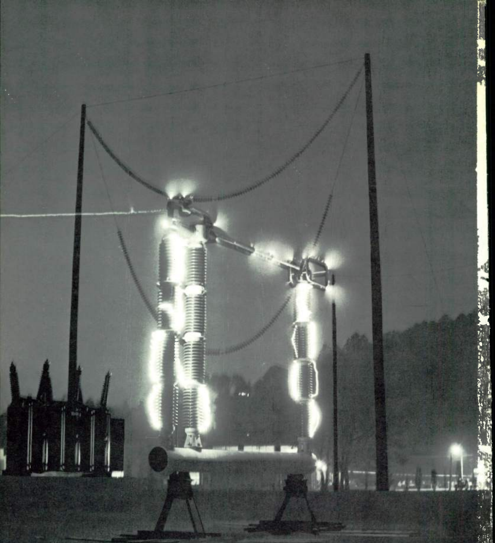
Multiple time exposures (note the star tracks) were used to obtain this dramatic photograph of a sixty-cycle flashover test of the 500-kv Type V-2 disconnect switch. The photograph was taken at the new Westinghouse EHV test center, where equipment ranging through the 1000-kv class can be tested fully.
