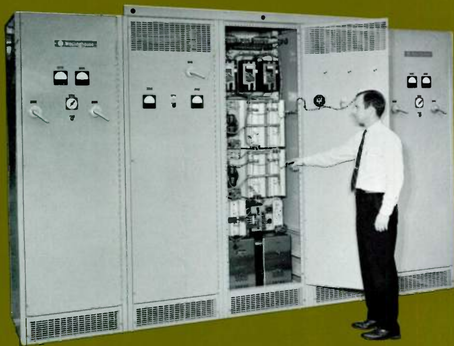
Two 10-kva inverters connected for use in parallel. Two separate battery chargers and batteries were applied in this system to give complete redundancy for supplying a critical load.
