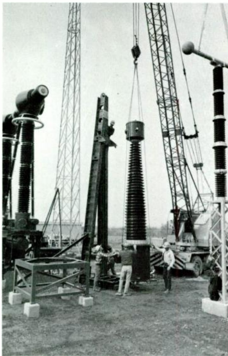
EHV current transformer is lifted from special truck in its protective cradle, set upright, separated from the cradle, and lifted into place on its foundation.
