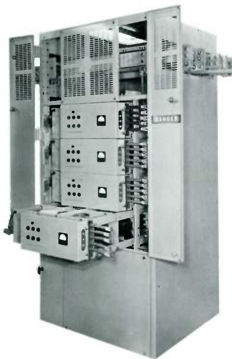
4—Thyristor cabinet includes up to four power cases and also a blower and the required number of gate-pulse amplifiers.
