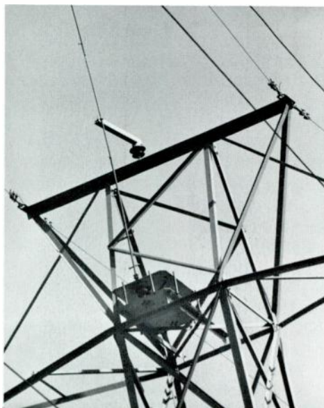
Typical kine-klydonograph installation atop a transmission line tower. Mast is visible at upper left. The instrument is located between the two parallel plates.
