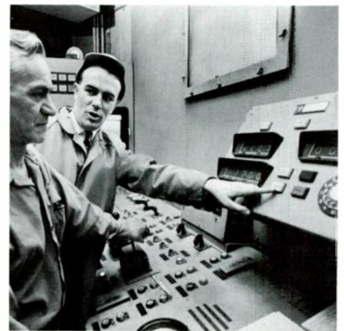
Control console in the operator's pulpit includes the control and monitoring devices that direct the charging, blowing, and other operations that produce a heat of steel. The dynamic control system enables the BOF to make steel faster, more economically, and with more uniformity.
