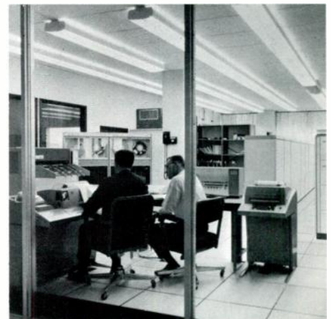
Packaged Computer Room
