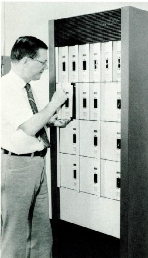
The new light dimmers are modular, made in several standard sizes to supply different amounts of lamp wattage. Each has a circuit breaker used as an on-off switch. Standardized cabinets hold as many dimmers as needed.
