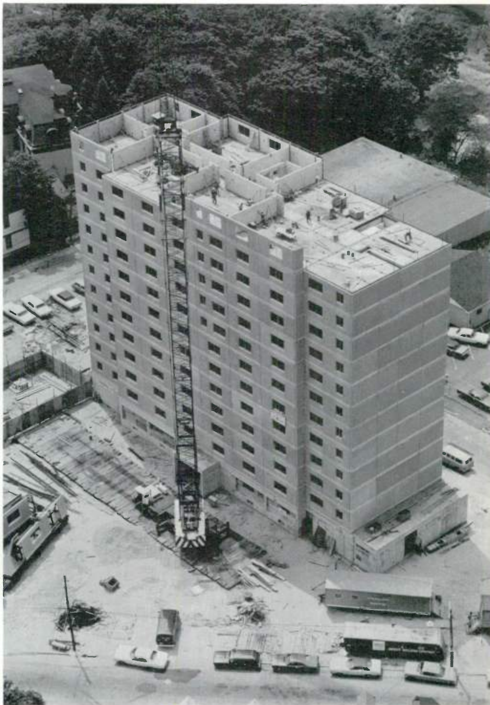
PROVIDENCE, Rhode Island—One of two 16-story Bison buildings for elderly housing is shown during erection. The photograph illustrates the floor-by-floor assembly of a Bison building, which permits interior work to proceed a few floors below the erection level.
