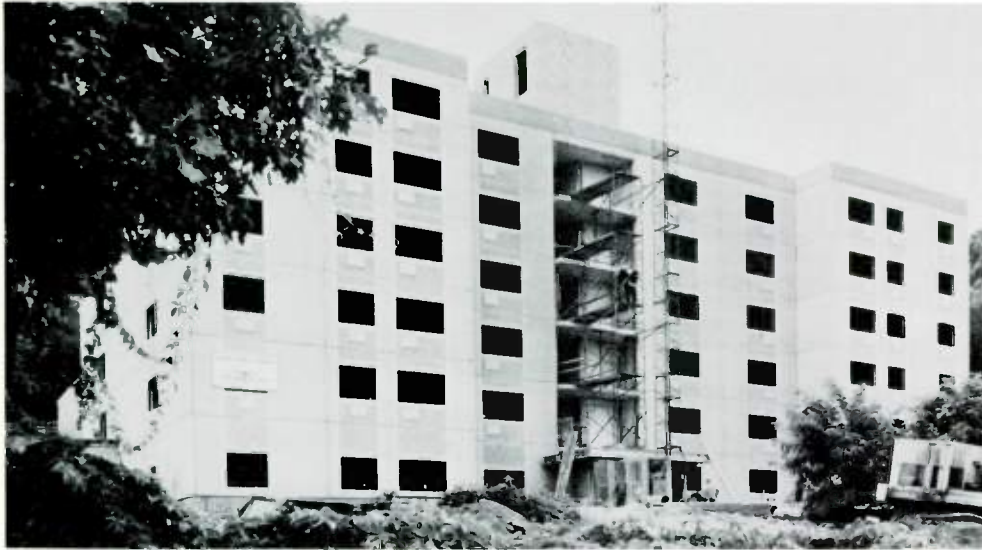
VERNON, Connecticut —(Left) The shell for this six-story 85-unit apartment building was completed in 6 weeks. The precast concrete components were manufactured at Blakeslee's Branford, Connecticut, plant, trucked to the site, and erected with an 85-ton crane. The building contains 181 exterior wall panels, 103 interior wall panels, 11 precast concrete stairways, and 194 precast prestressed concrete floor planks.
