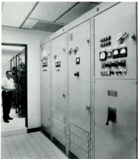
3—This 75-kVA UPS system protects a data-processing computer at San Diego Federal Savings and Loan. Its battery room can be seen in the background.
