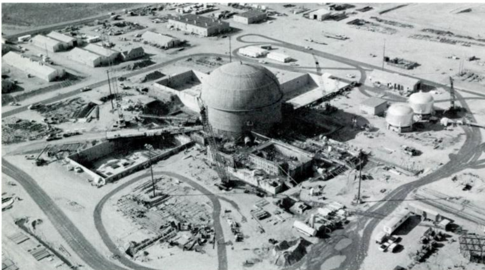
FFTF containment vessel is receiving final construction touches while other buildings go up.
