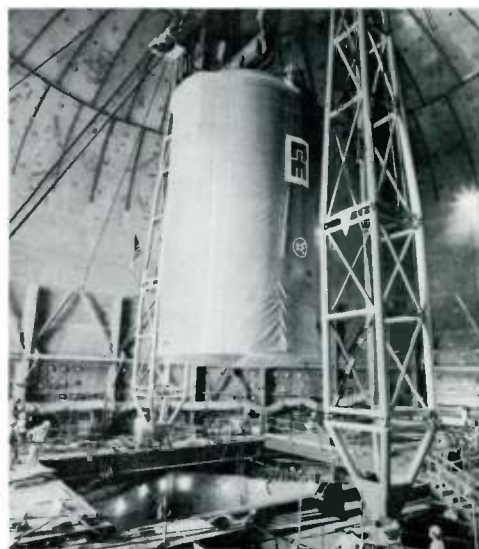
Workmen lower the Fast Flux Test Facility's guard vessel into the reactor cavity. The guard vessel is one of many safety features built into the FFTF, which will be used to test fuels and components for the nation's liquid-metal fast breeder reactors.
