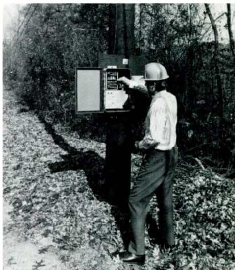
3—A prototype transmitter/receiver for use in feeder automation is also installed on the Carolina Power & Light Company system. It performs much the same functions as the home unit, but it performs them on the high-voltage part of the distribution system.
