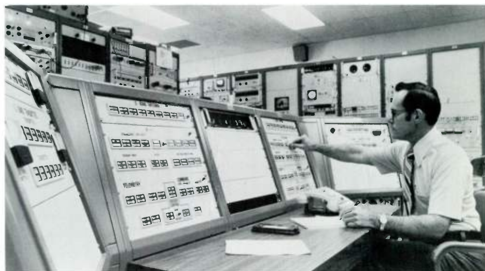
This equipment provides the means for controlling SMS satellites and for acquiring, synchronizing, and stretching the data received from them. It is located at NOAA's Command and Data Acquisition Station.
