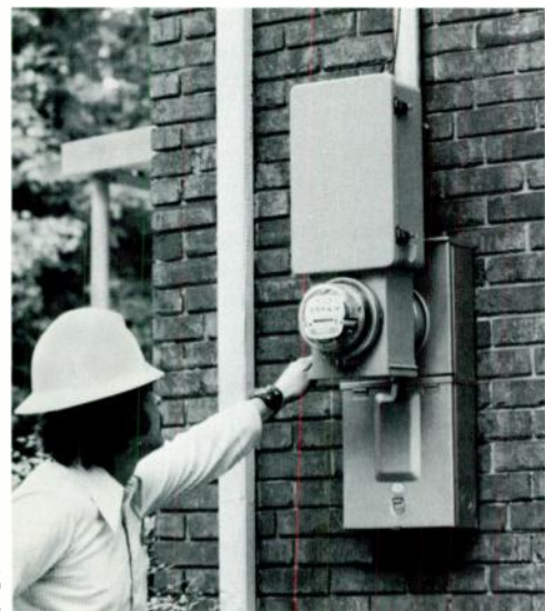
2—This prototype home transmitter/receiver for distribution-line carrier communications, shown here installed on the residence of a Carolina Power & Light Company customer, is part of the equipment used for field trials. It performs such functions as automatic meter reading, selective load control, voltage continuity monitoring, and remote service connect/disconnect.
