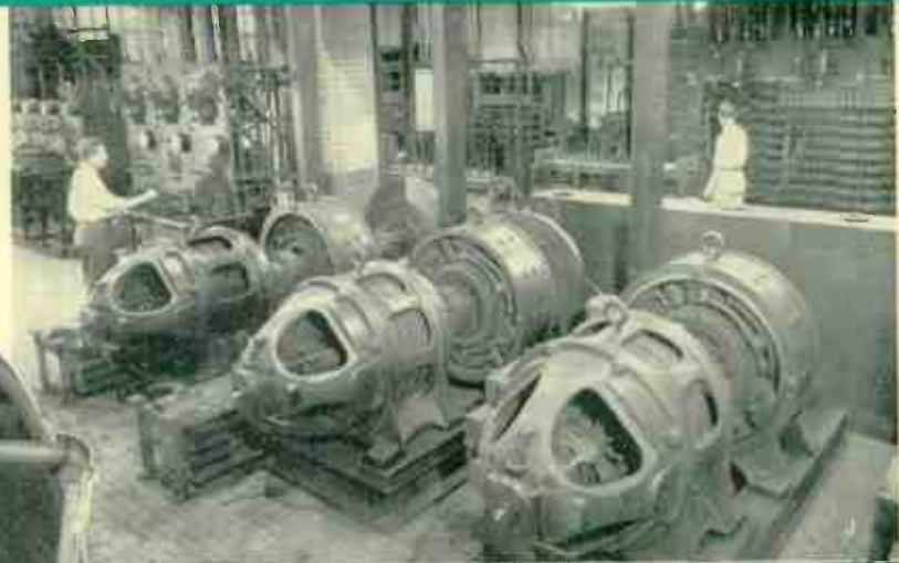
J —The flywheel motor-generator sets and panels in the rear with capacitors provide an artificial transmission line for stability studies. K —This device is a locomotive, or so it appears to the mercury-arc rectifiers given a shake test to determine their action in rail service.
