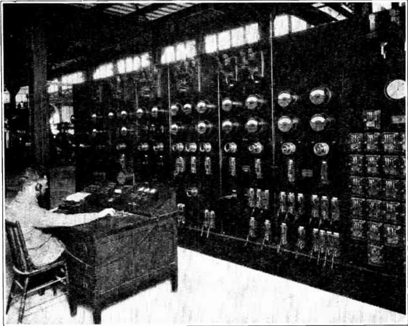
Fig. 13—Main Control Panel, Rocky Point Single Side Band Eliminator Carrier Transmitter
