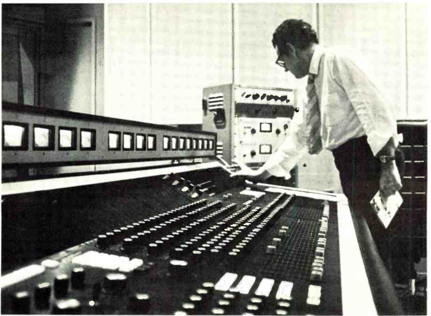
Now happily installed and busy, the Audio Designs console dominates the control room of Mercury's Studio A.
