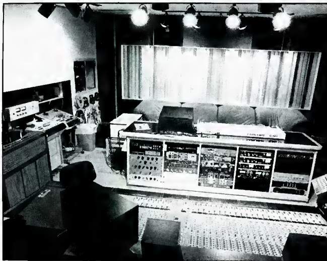
Figure 5C. Rear view at Chicago Trax Recording, Acoustical consultant Doug Jones, Electro-Acoustic Systems, Inc. The LFD can be seen behind the RPG cluster.
