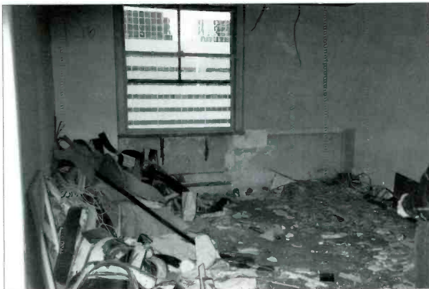
Figure 1. Demolition time at Howard Schwartz Recording. Raw space after everything is out.
