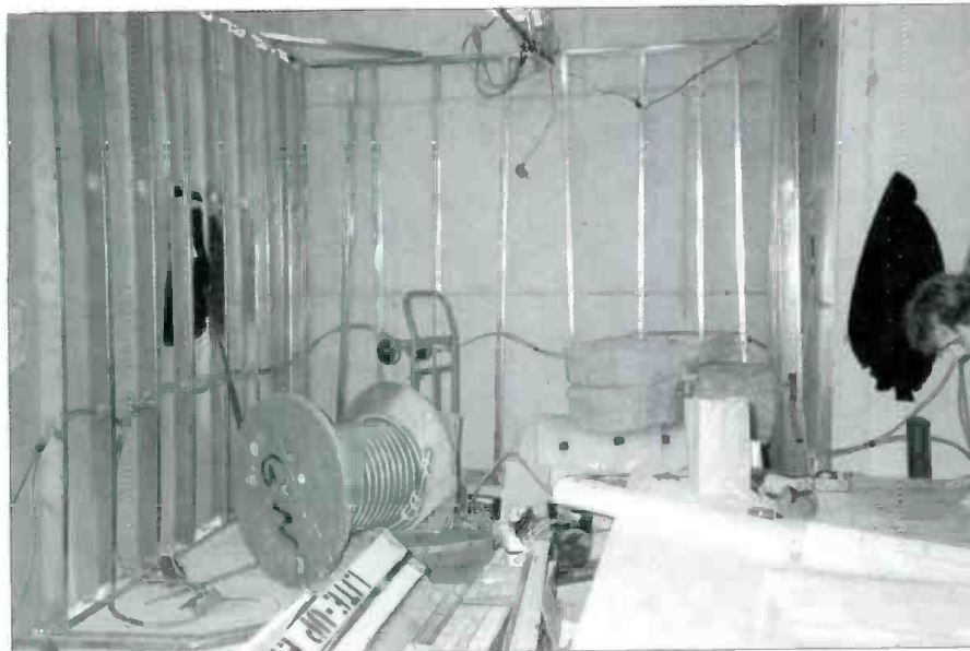
Figure 2. Some of the formers and wiring in the still raw space.
