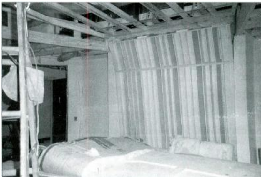
Figure 4. RPG diffusers are in place, but will their effectiveness be altered by being painted?
