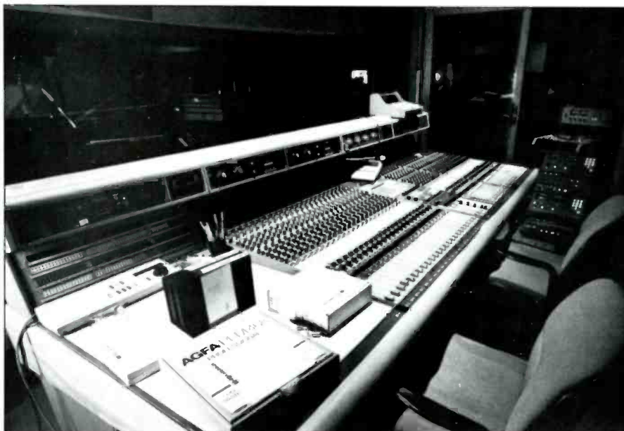
Figure 7. Streeterville studio 1 has a Neve 8128 48-channel with NECAM and a 4-machine lock-up.
