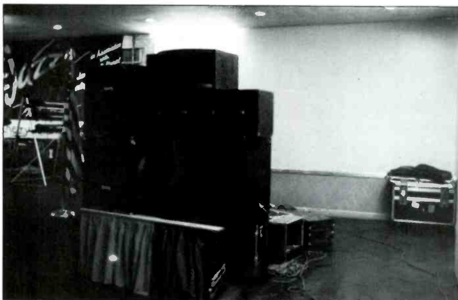
Figure 7. The house-right PA stack. Wyndham Hotel ballroom, Kingston, Jamaica. PA amplifier racks are visible behind and next to the PA.
