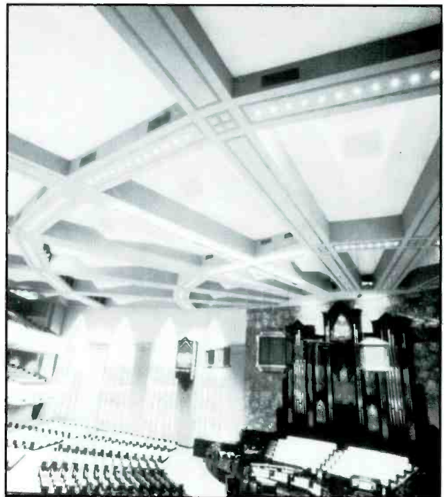
Figure 4. Additional loudspeaker arrays are ceiling-mounted in the sanctuary to provide balcony area reinforcement.
