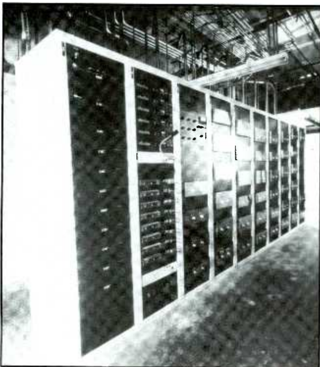
Figure 1. Housed in Atlas/Soundolier racks, 26 Crown PS-400 and 15 PS-200 amps send power to the main sanctuary.
