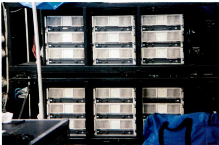
Figure 4. Traveling carts for the amplifier racks
