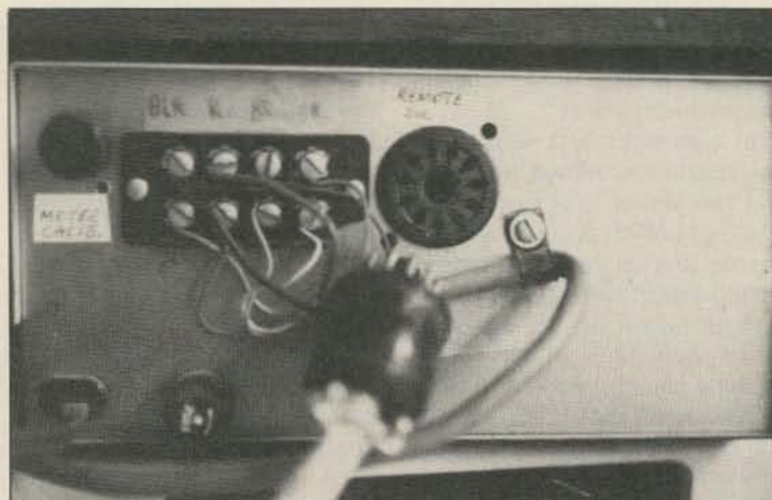
Photo B. CDR rear panel. The relocated calibration pot is at upper left.
