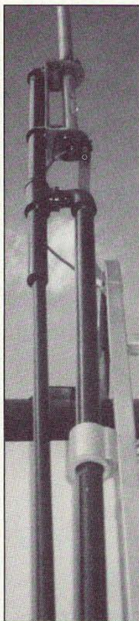
Photo A. Close-up of the antenna mount.
