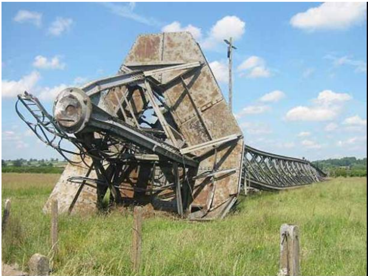
One of the masts lying on the ground the following morning (Photo copyright BT)
