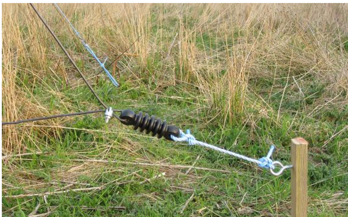
Figure 4: Photograph of loop support showing insulator and cable clamp.
