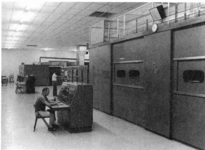
Fig. 1-5 This is Transmitter Hall at Trans-World Radio in the sunny Netherlands Antilles. TWR's huge 500kW (800kHz) AM broadcast transmitter is shown being monitored from the foreground console. A 260kW shortwave broadcast transmitter is being adjusted in the background. (TWR photo)
