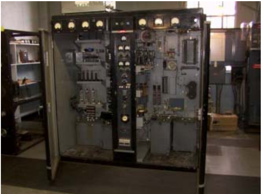
Inside one of the transmitter cabinets All photographs courtesy of Yuri Muzyka, Auckland
