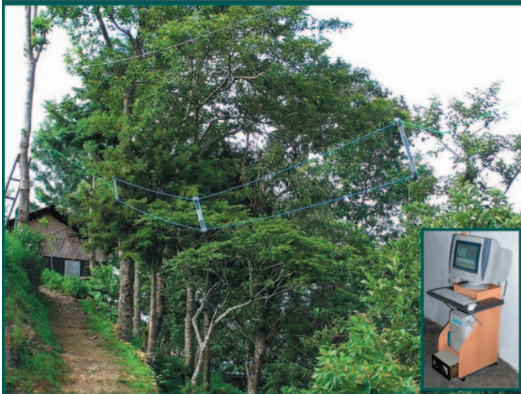
Photo: T2F Dipole Antenna for Remote Monitoring System, TWR- India, Kohima, Nagaland
